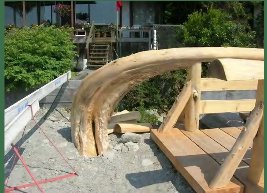
Bridge built with salvaged urban wood at the Lawson Creek Estuary in Ambleside
