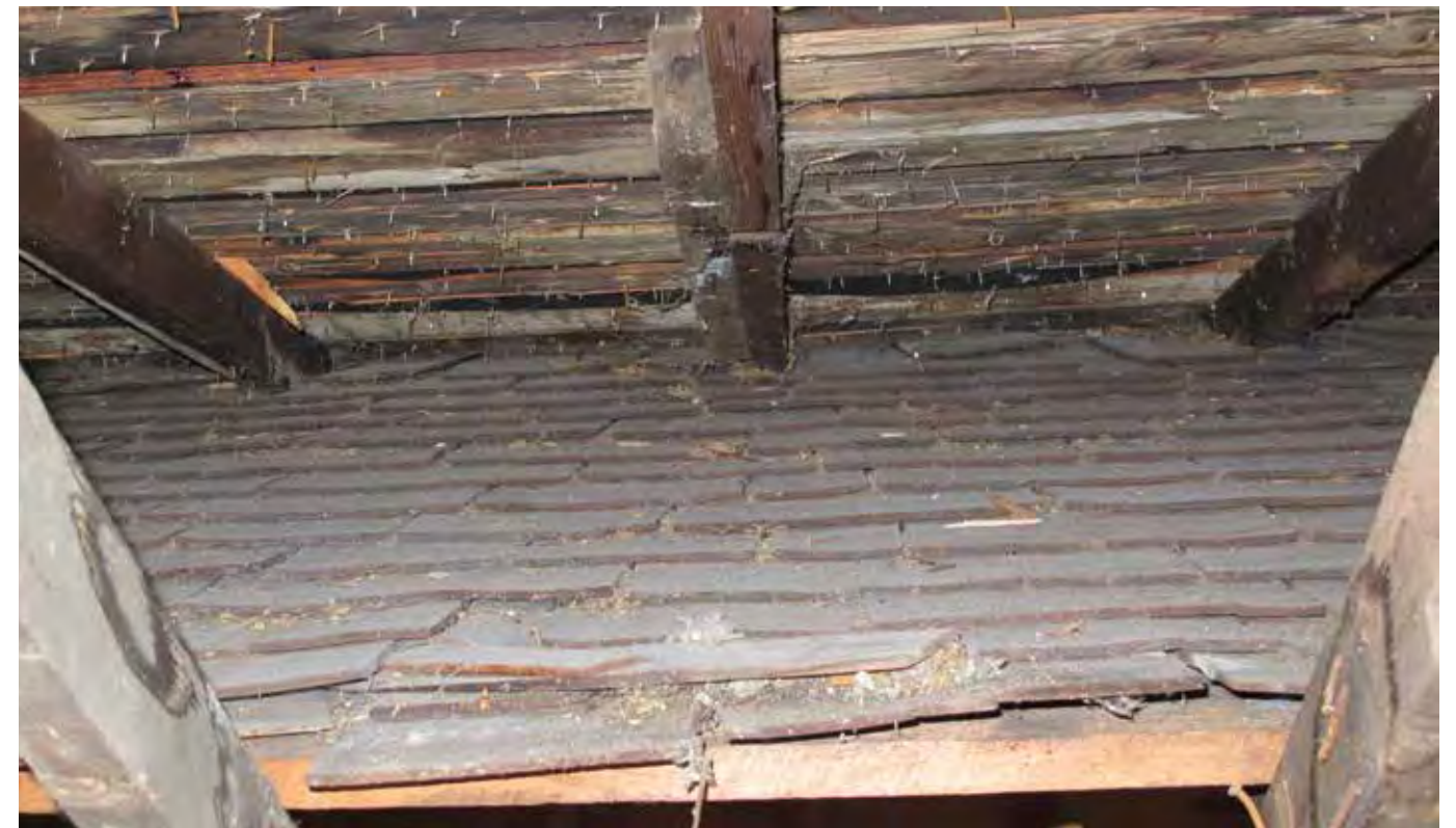
Evidence of chimney fire in the East Gables.
