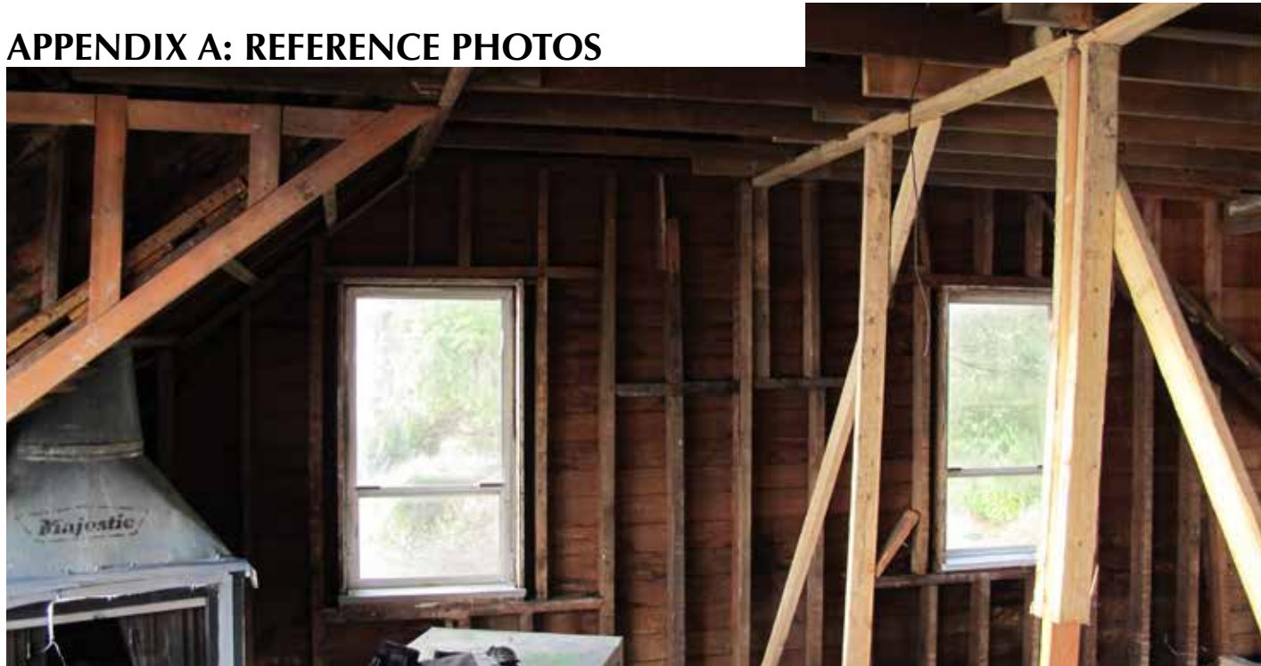
None of the window frames or assemblies have survived, but the window openings are clearly evident on the second floor and provide measurements for how the windows can be restored. Original double-hung configuration as per archival photos.
