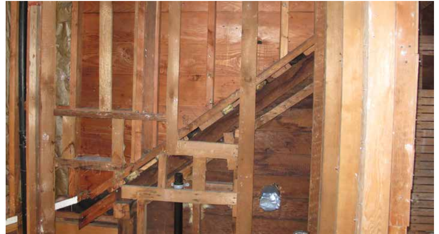
Although the roof framing has been cut out in several locations, virtually all of the planking that formed the exterior soffits were left in place, and can be traced on the east and west sides of the house.
