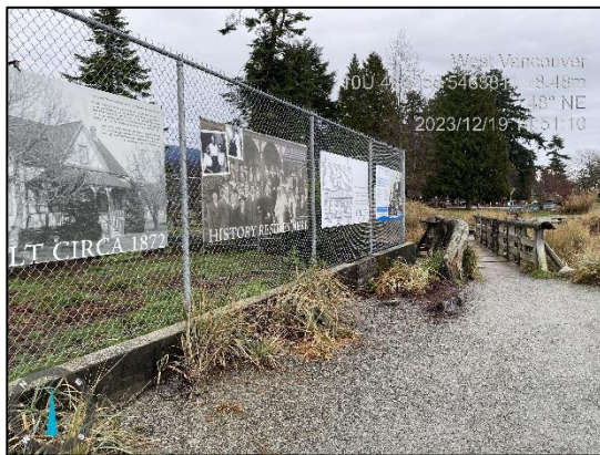
Photo 3: View of the concrete retaining wall separating the Property from the Centennial Seawalk.
