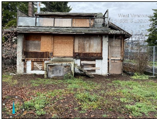
Photo 1: View of the Navy Jack house with chainlink fence surrounding the site.
