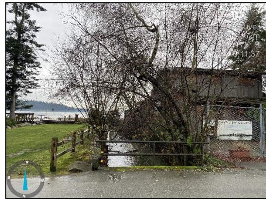
Photo 2: View of the concrete flume with Lawson Creek, adjacent to the house.
