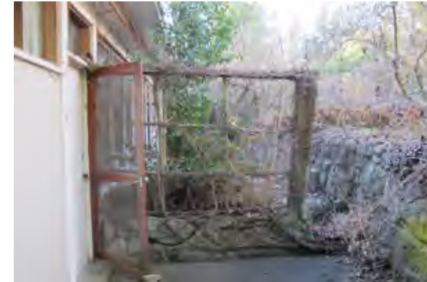
Image of Binning garden in it's current state (2017) (wood trellis to be replaced & stone wall to be retained / repaired as required)
