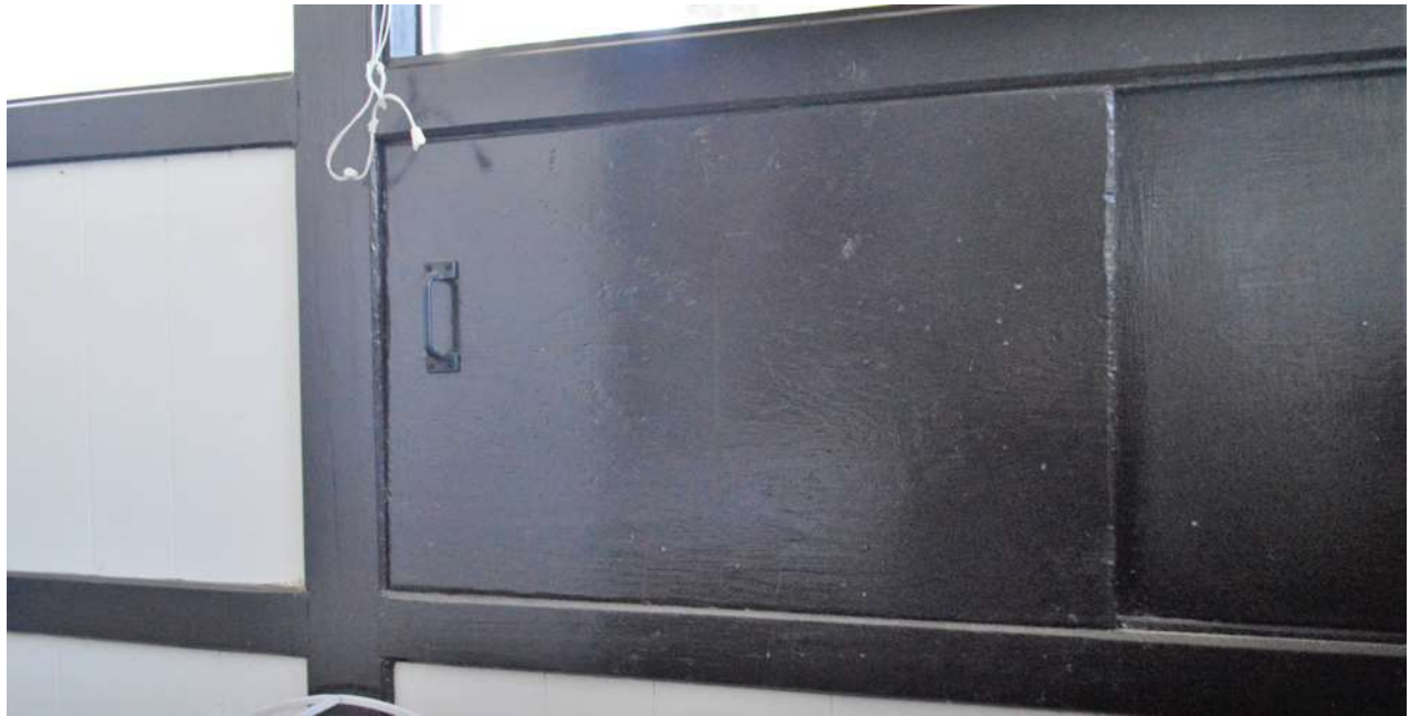
Figure 100: Sliding panel door ventilator
