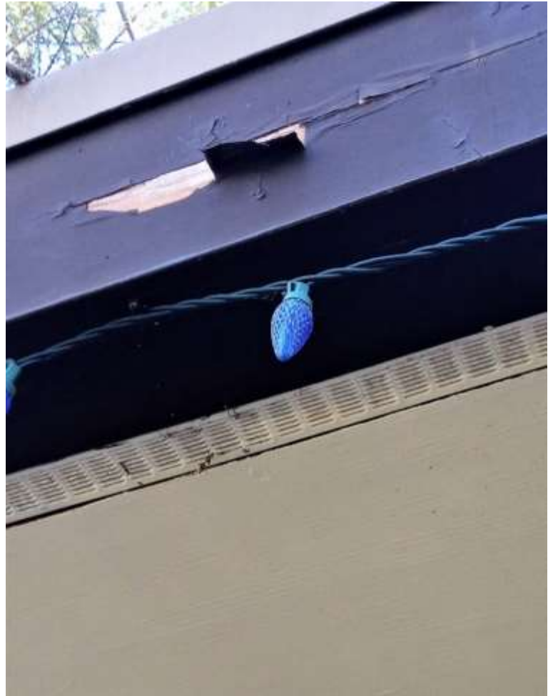
Figure 95: Roof soffit vents and paint peeling at fascia
