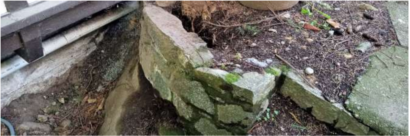
Figure 74: North side terrace stone steps edge
