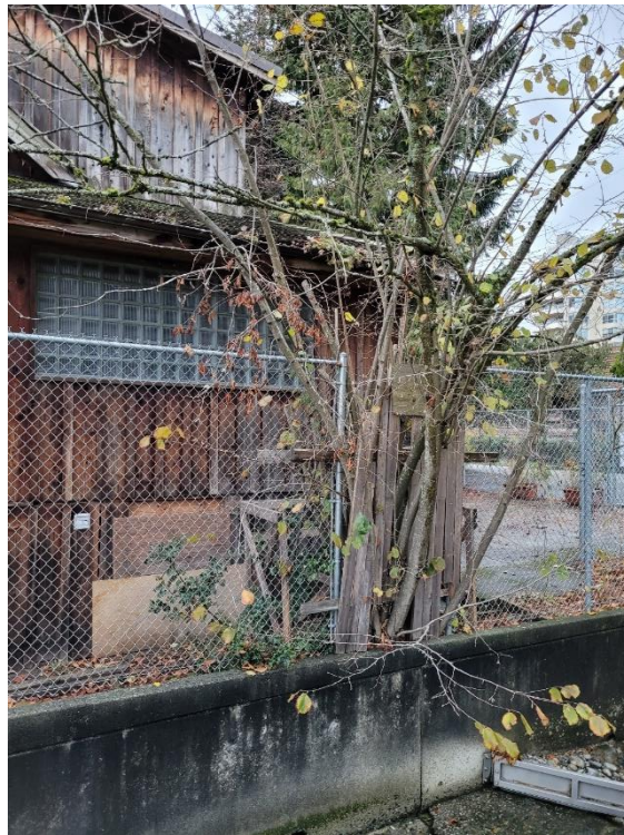
Photo 4. Tree #38, growing in retaining wall.
