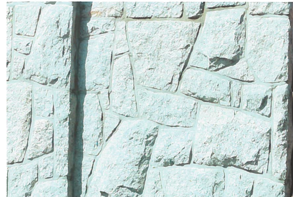
12 Stone wall facing and garden walls will be in white "Ambleside" granite as supplied by Northwest Landscape Supply in full thickness veneer, matchint the neighbouring house at 4727 Pilot House Road.
