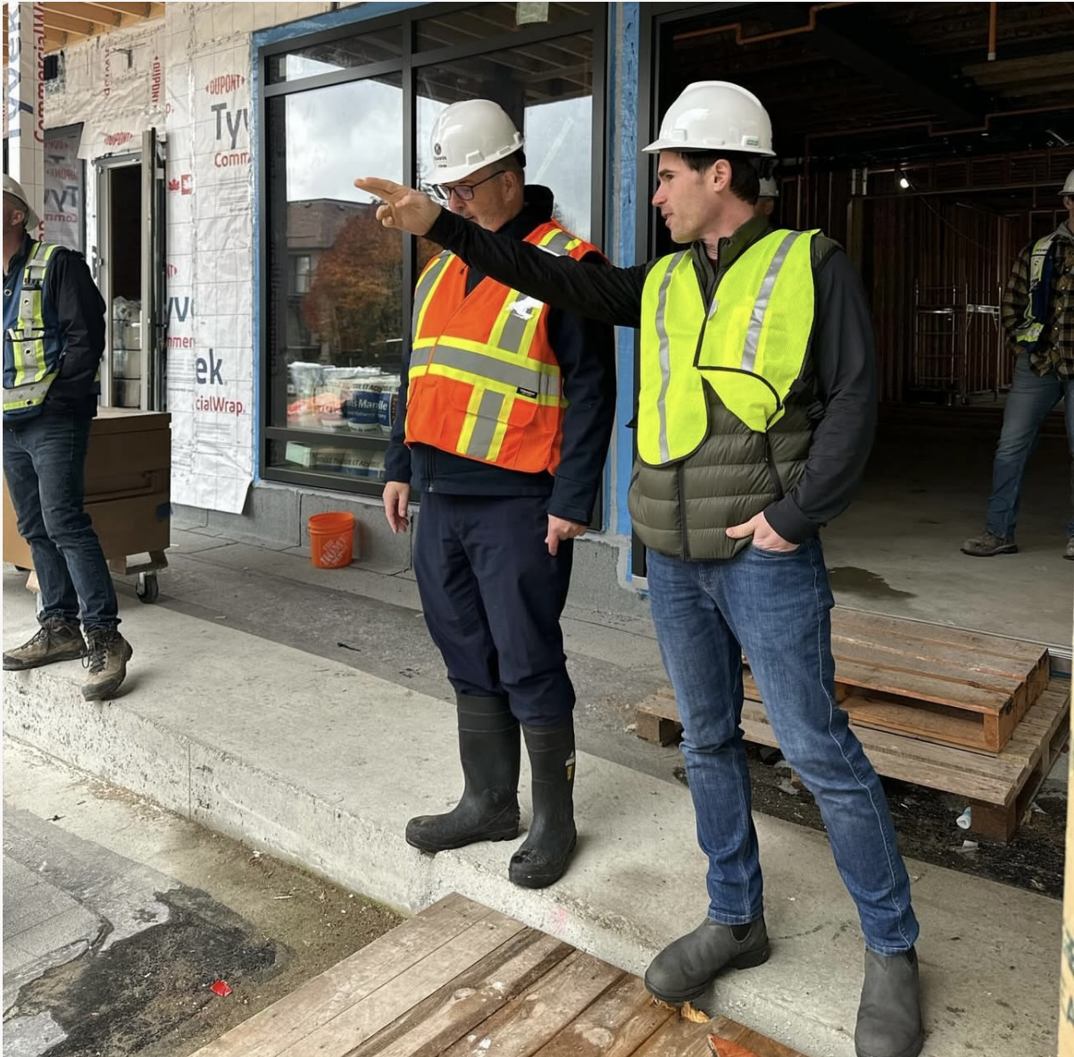
Site visit to see progress on the Kiwaniis Village West affordable housing project in West Vancouver, funded by the federal government
