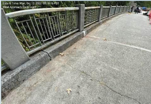
66. Cracking on Asphalt Wearing Surface at West Approach Deck Joint, Typ.
