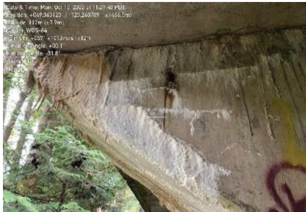
60. Efflorescence on Deck Soffit of West Abutment
