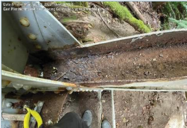
50. 4mm Section Loss at Northwest Base of West Pier
