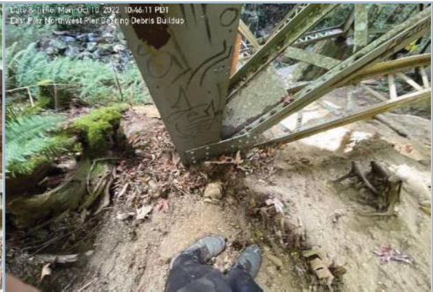
51. Debris Accumulation at Pier Northwest Column Base of East Pier
