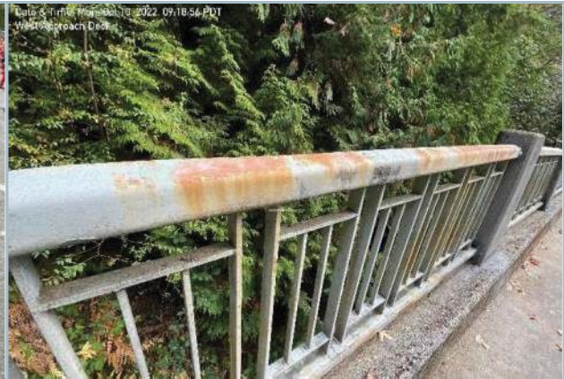
67. Localized Inconsequential Surface Corrosion on Northwest Railing, Typ.
