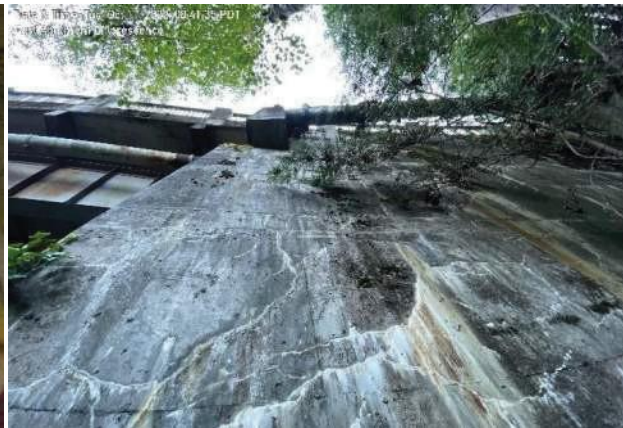
061. Extensive Efflorescence at East Abutment Wing Wall
