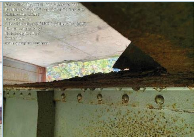
403. Steel Delamination and Deposit Accumulation at South Girder, Typ.
