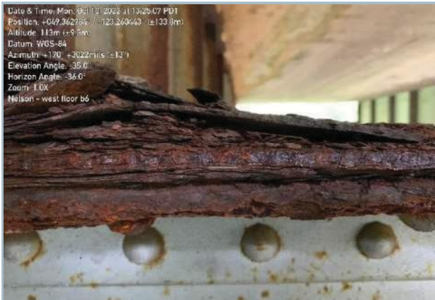
40. Accelerated Uniform Corrosion on Top Flange of Floor Beam 5, Typ.
