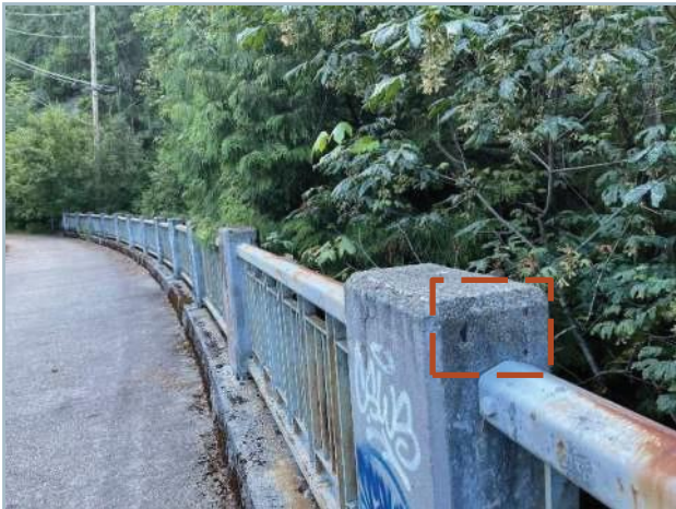
68. Localized Exposed Reinforcing on Deck Parapet at Midspan
