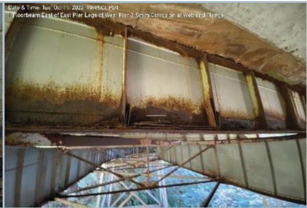
39. 3-5mm Section Loss on Bottom Flange of Floor Beam 9 (Note: Top Flange Corrosion, Typ.)
