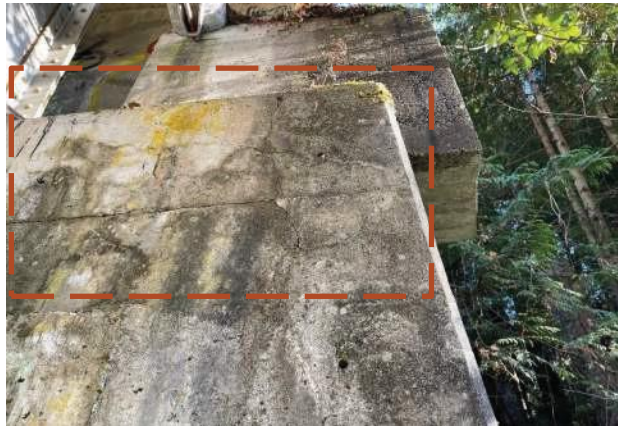
062. Extensive Cracking at East Abutment Side Wall
