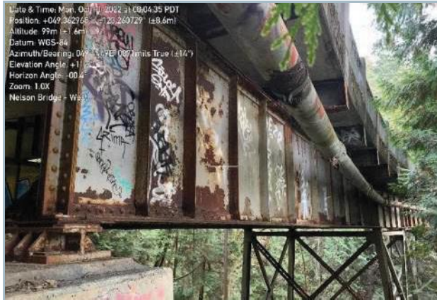
48. South Girder Bottom Flange Corrosion, Typ.
