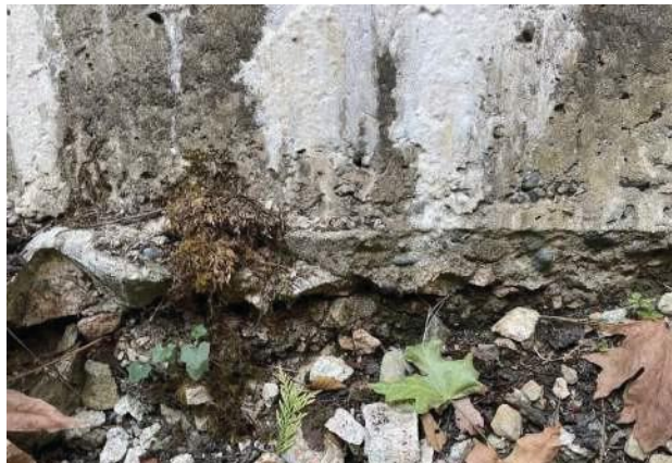
64. Undermining and Aggregate Exposure East Abutment Wing Wall
