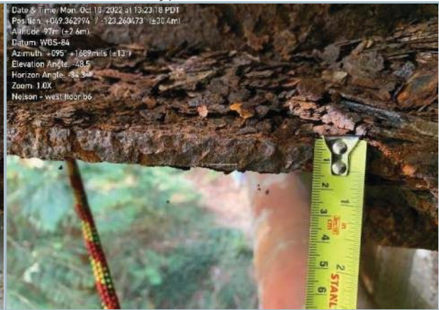
045. 3-5mm Section Loss at Bottom Flange of Floor Beam 6
