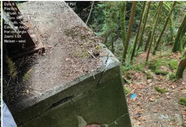
063. Cracking and Separation at Southeast Pedestal of West Pier, Typ.
