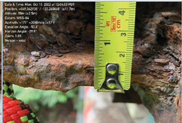
41. 3-5 Section Loss at Bottom Flange of Floor Beam 5 Below Expansion Joint
