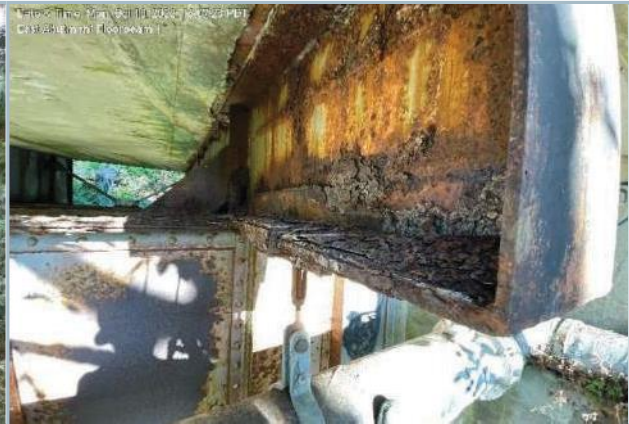
049. Accelerated Corrosion and Deposit Attack on Floor Beam 2
