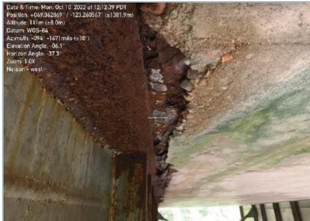
46. Top Flange Corrosion and Spalling of Deck Soffit at Floor Beam 14
