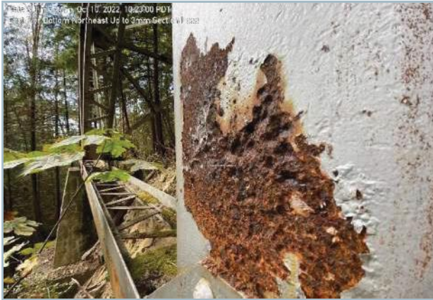
36. Pitting Corrosion with ~3mm Section Loss at Bottom of Northeast Pier
