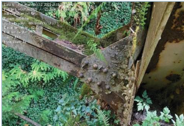
52. Vegetation Growth on East Pier Connection, Typ.
