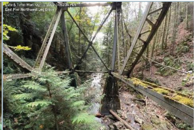
053. Debris Accumulation on Pier Truss Elements of East Pier
