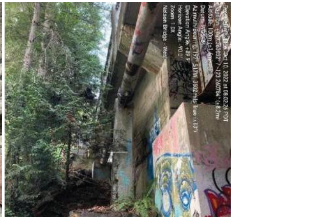
65. Undermining and Aggregate Exposure West Abutment Wing Wall
