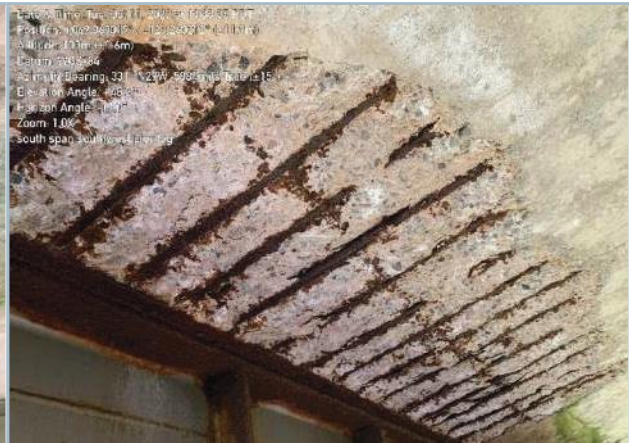
47. Exposed Reinforcing Section of Deck Soffit at Floor Beam 15
