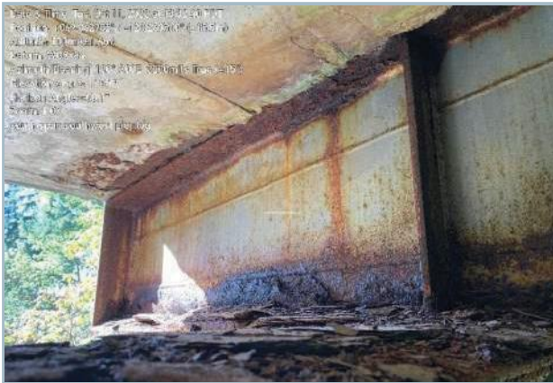
38. Accelerated Uniform Corrosion at Bottom Flange of Floor Beam 5
