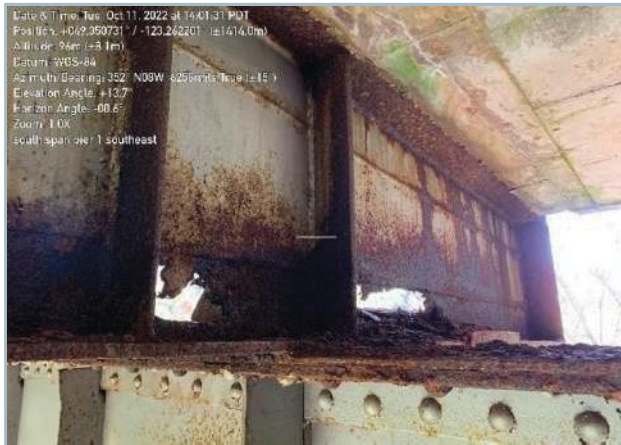
42. Complete Section Loss at Floor Beam 7
