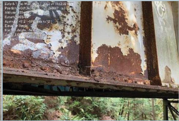
37. Deposit Attack and Accumulation on Bottom Flange of South Girder, Typ. (Note: Deterioration of Rivets)
