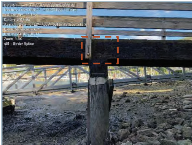
036. Unbalanced Longitudinal Beam Bearing Seat
