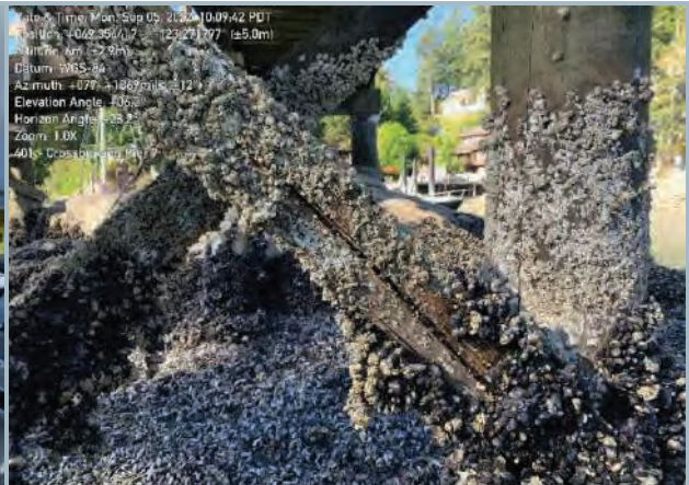
027. Decaying Timber Brace at Pier, Typ.
