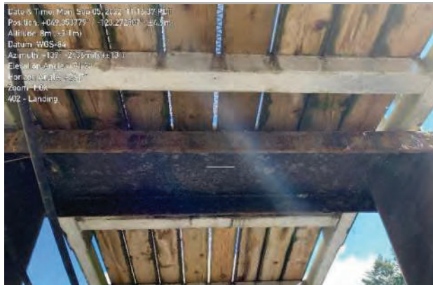
018. Minor Surface Corrosion of Pier Cap
