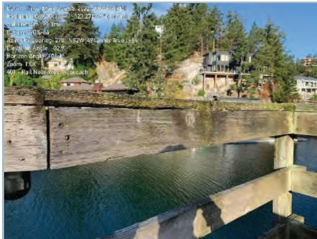
030. Localized Lifting of Decaying Top-rail, Typ.
