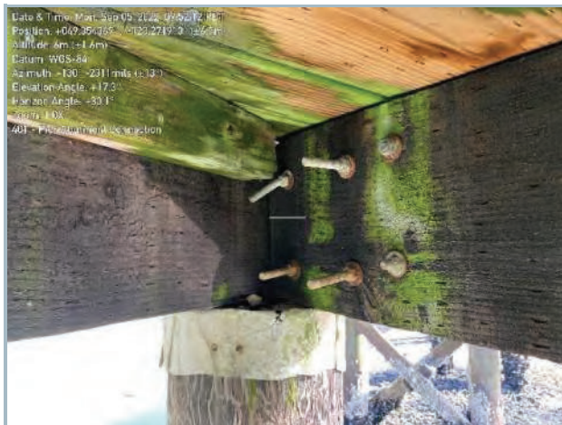
038. Inadequate Placement of Anchors at Bedrock Pier
