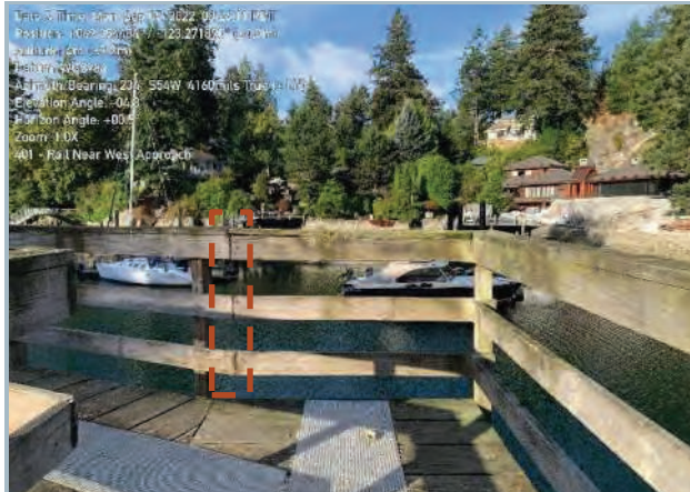
024. Vertically Unsupported Timber Splice at Bedrock Pier
