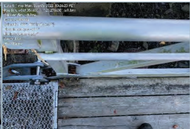
012. Debris Accumulation at Rail Truss Base
