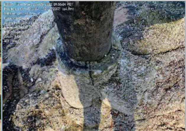
025. Cracked Concrete Pedestal at Bedrock Pier
