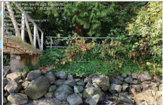
019. Minor Undermining at Northwest Section of West Backwall
