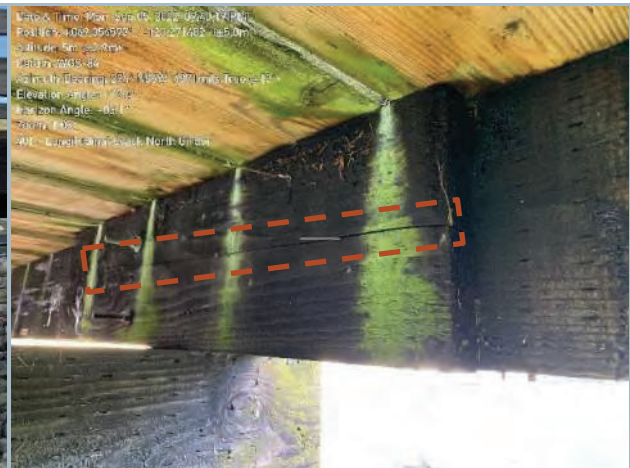
037. Full Longitudinal Splitting of Timber Splice
