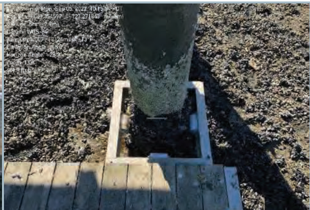
010. Dock Restraint Timber Pier Connection
