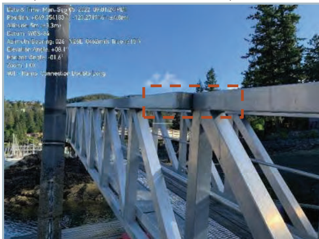
017. Extended Gangway Connection
