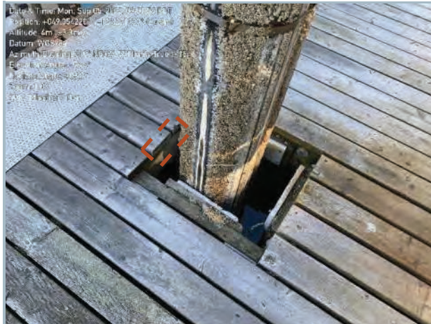
032. Timber Pier Dock Restraint Missing Teflon Bumper
