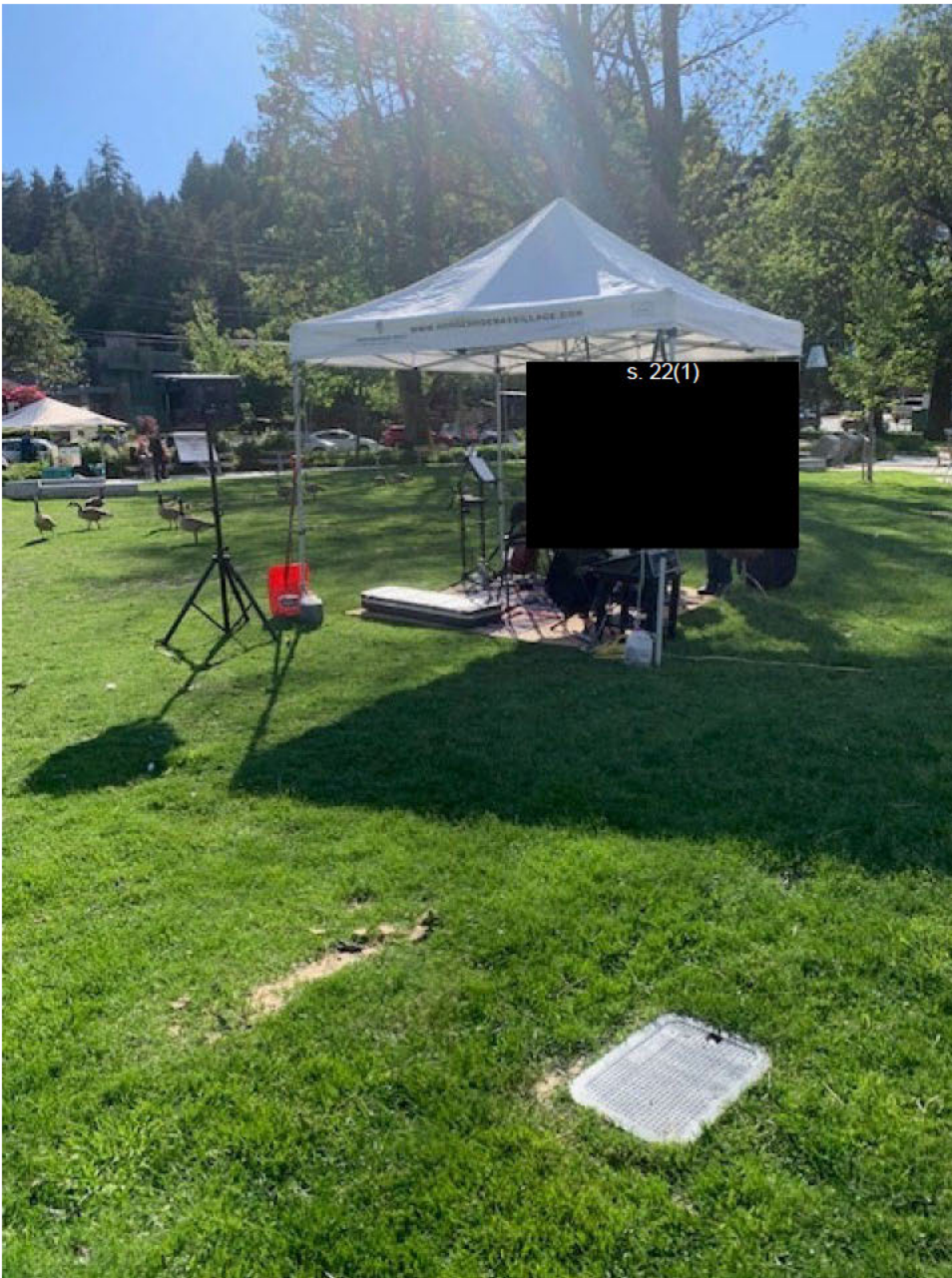
This electrical panel was not connected when the park was revitalized. A generator had to be rented last minute on a busy day!
