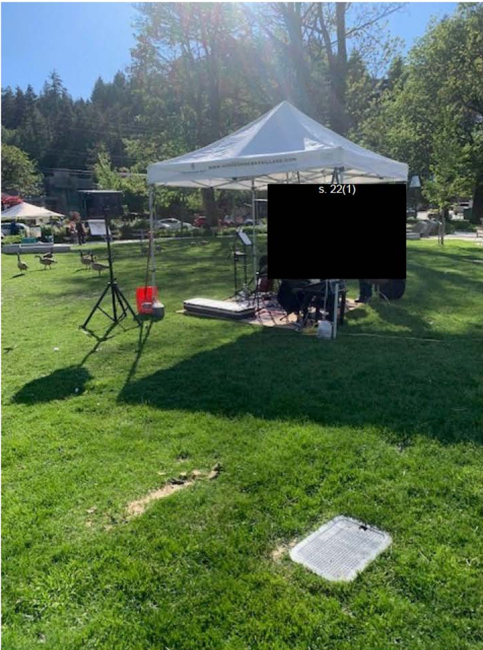
This electrical panel was not connected when the park was revitalized. A generator had to be rented last minute on a busy day!
