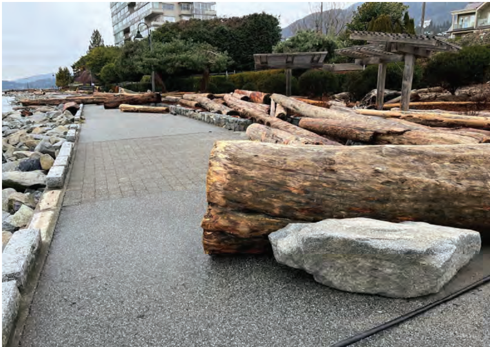
Figure 3-6. Deposited debris and dislodged armour rocks on the Centennial shoreline following the January 7th, 2022 storm – facing west.
