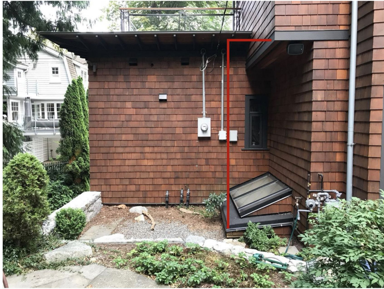
Photo #1 – Area of addition (33.13 ft 2 ) – foundation around skylight (7ft X 4ft) and below upper floor living space.
