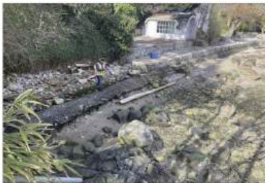
Photograph No. 2 Looking North along the shore of the properties. Note exposed concrete encased sanitary line where surveyor is standing.
