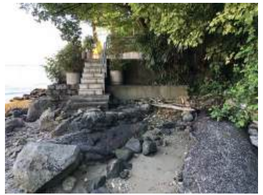
VIEW LOOKING SOUTH THE PORTION IN FRONT OF THE PROJECT SITE IS HEAVILY ERODED CREATING A SIGNIFICANT GRADE DIFFERENCE BETWEEN THE SOUTH NEIGHBOUR TERRACES AND EXPOSING THE SEWER PIPE INFRASTRUCTURE VISIBLE IN THE RIGHT SIDE OF THE IMAGE
