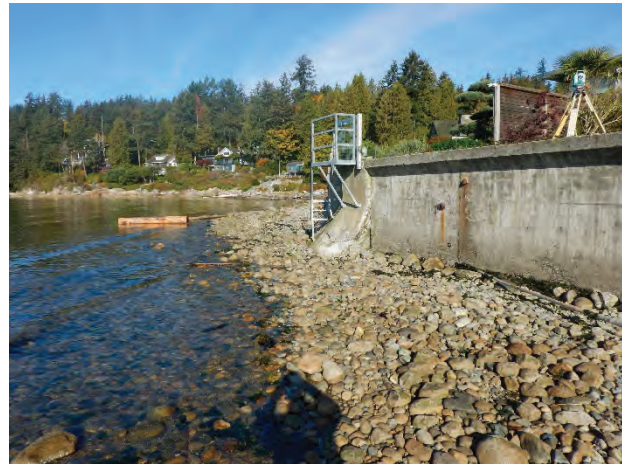
Photo 4. Potential scour near the wall, looking east of the property
