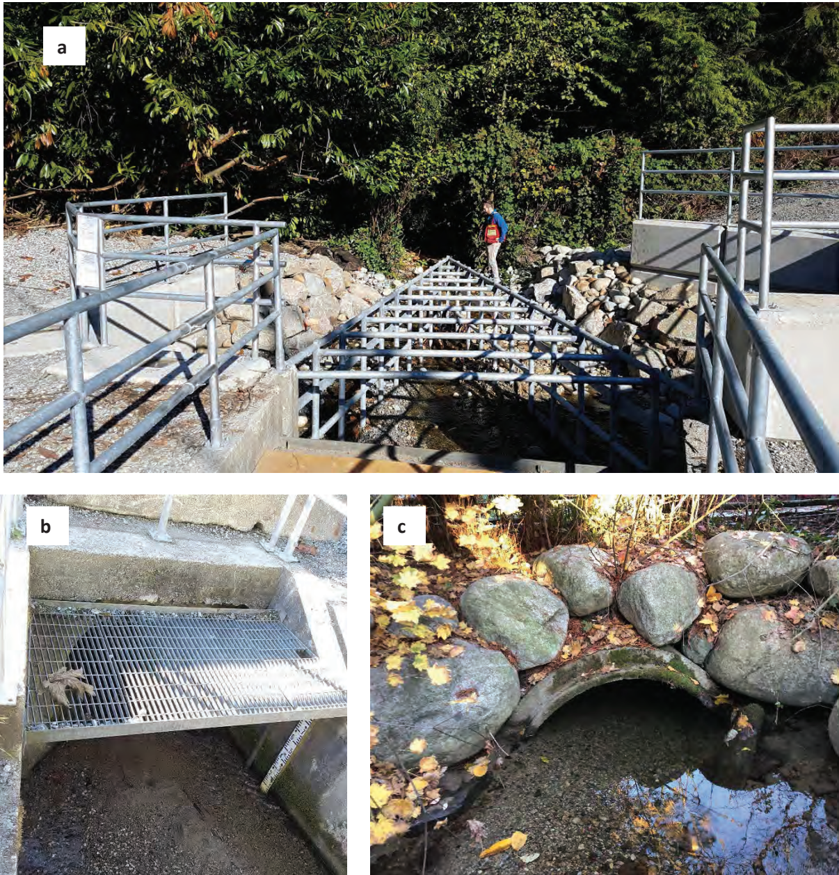
Figure B.2. Willow Creek photos (a: new trash rack at inlet, b: culvert inlet, c: outlet)
