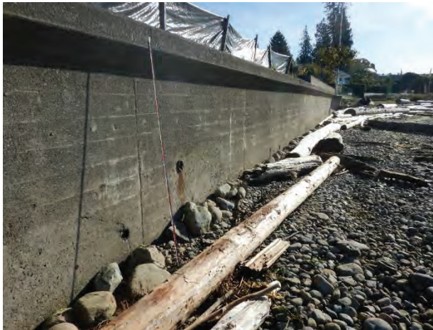
Photo 3. Potential scour near the wall, looking west of the property
