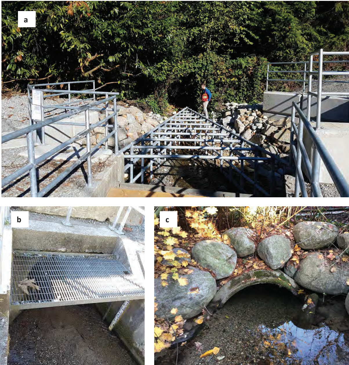
Figure B.2. Willow Creek photos (a: new trash rack at inlet, b: culvert inlet, c: outlet)
