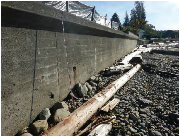
Photo 3. Potential scour near the wall, looking west of the property
