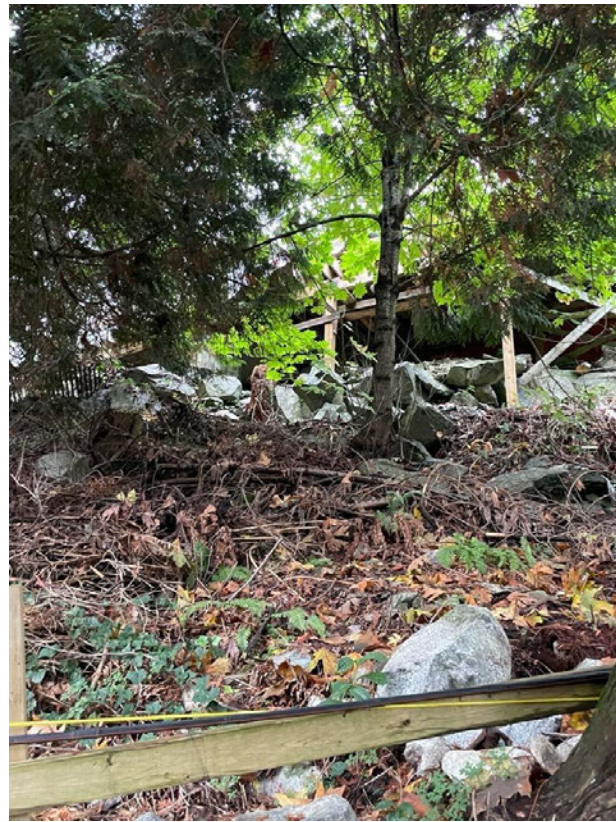
Figure 2: Insufficient Footings and Supports
