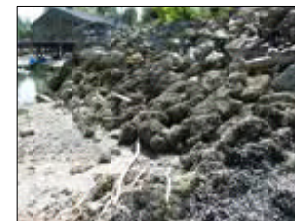
Image 2. Rip rap conditions found along northern face of parking area.
