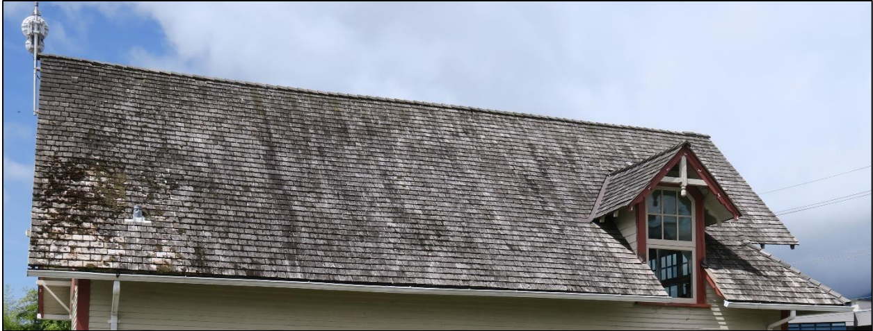
Fig. 17: Eastern side view of the Ferry Building Gallery, 2020, illustrating the current state of the roofing. (Source: Ehman)
