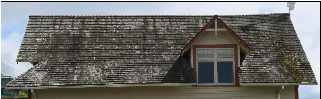
Fig. 18: Western side view of the Ferry Building Gallery, 2020, illustrating the current state of the roofing. (Source: Ehman)
