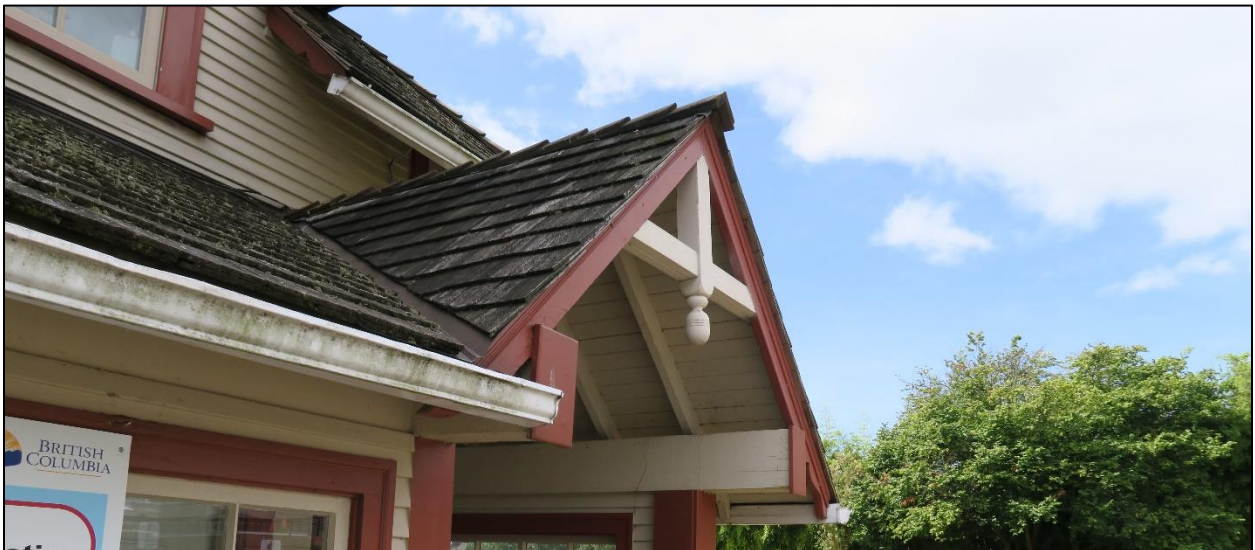
Fig. 19: Partial front view of the Ferry Building Gallery, 2020, illustrating the state of the front roofing and some of the eaves. (Source: Ehman)
