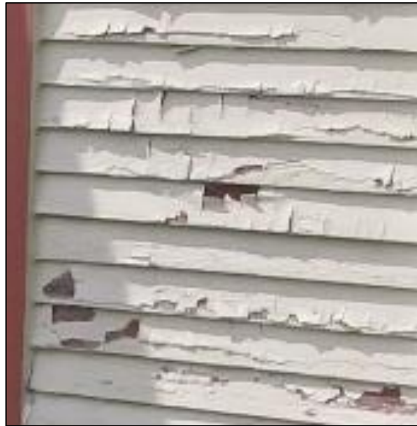
Fig. 23b: Detail shot of the eastern side of the Ferry Building Gallery, 2020, illustrating the areas of peeling paint. Note this also reveals the earlier, inverse paint scheme with a darker red for the main body colour. (Source: Ehman)
