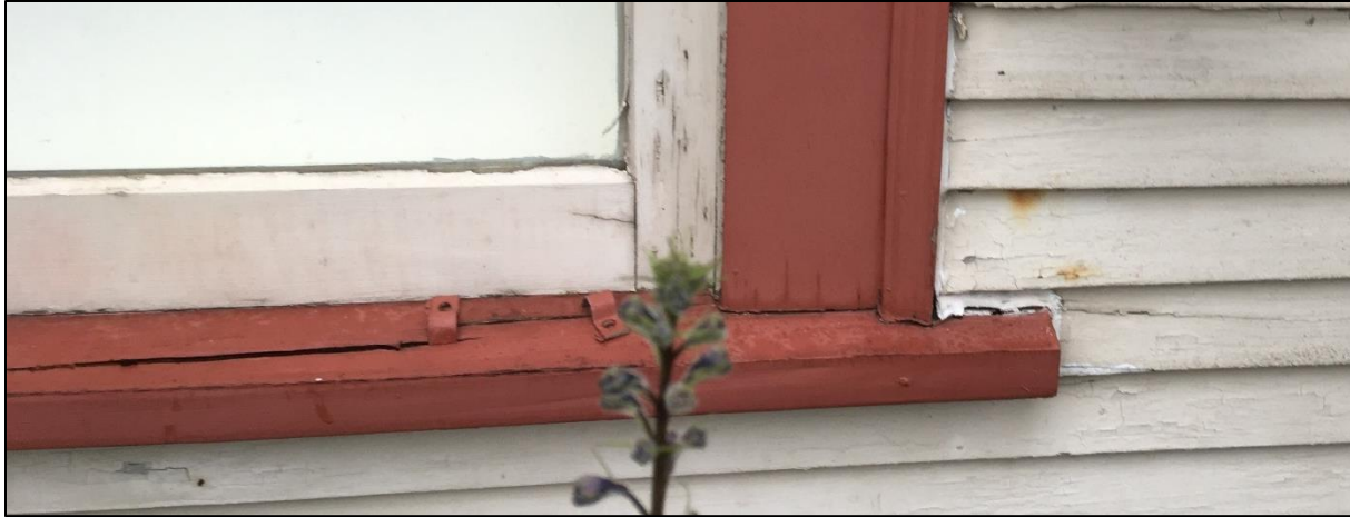
Fig. 22: Detail shot of one of the eastern windowsills and trims, showing signs of deterioration, including a large crack in its sill. (Source: Ehman)
