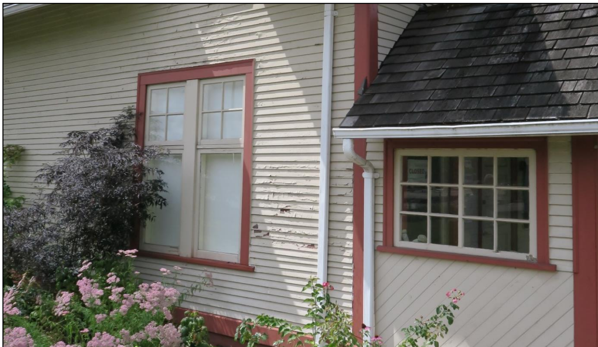
Fig. 23a: The eastern side of the Ferry Building Gallery, 2020, illustrating the condition of the siding, in particular showing areas with peeling paint (a detail shot of which is shown in Fig. 23b below). (Source: Ehman)
