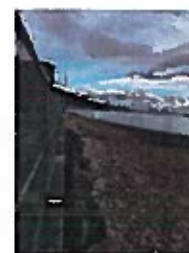
SOUTH EAST FORESHORE ENCROACHMENT
