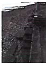
SOUTH EAST FORESHORE ENCROACHMENT
