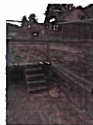
SOUTH EAST FORESHORE ENCROACHMENT
