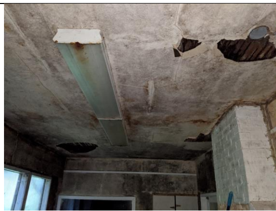
Photo 4: Upper floor ceiling showing significant water ingress
