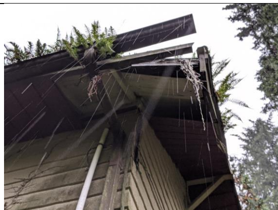
Photo 6: Damaged roof overhang at northwest corner of the building.
