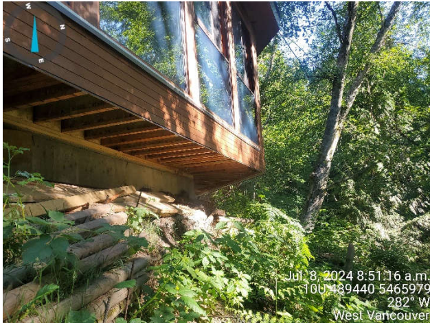
Photo 1: View of north side of the unpermitted building overhanging ToB.
