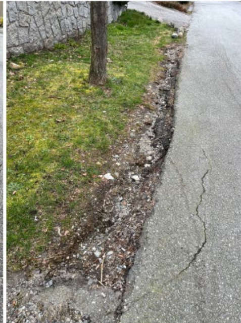
Damaged boulevard from vehicles parking on boulevard is causing erosion.
