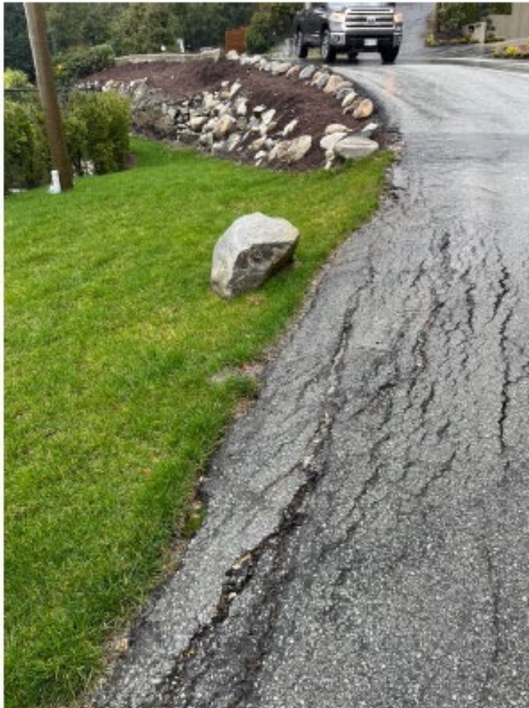
Vehicles parking close to road edge are damaging asphalt road edge.
