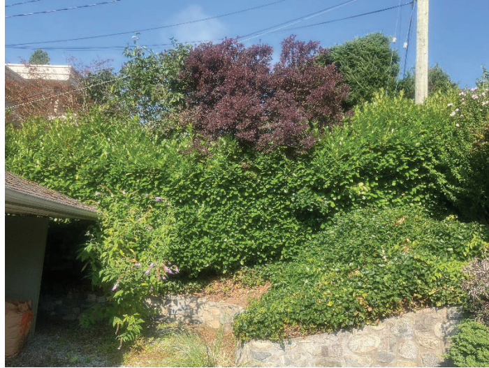
Photo 7. The upper section of hedge1 is growing within the bounds of a retaining wall on the West side of the property
