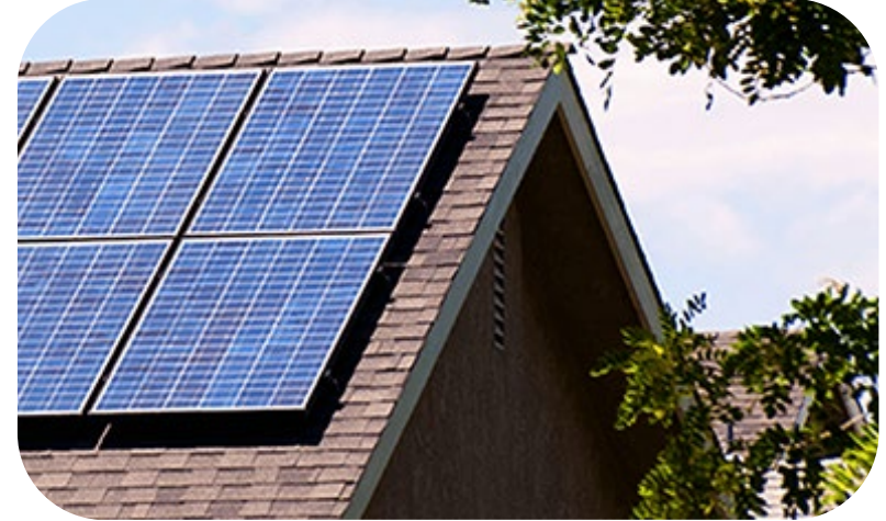
BCHydro.com – Solar panels
