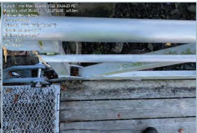
012. Debris Accumulation at Rail Truss Base
