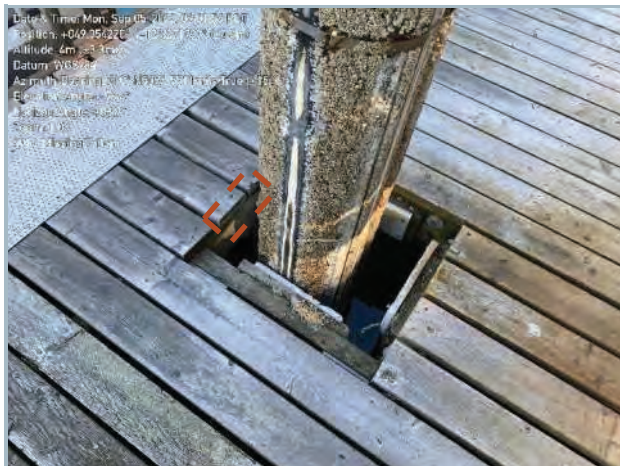
032. Timber Pier Dock Restraint Missing Teflon Bumper
