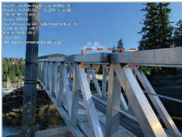
017. Extended Gangway Connection
