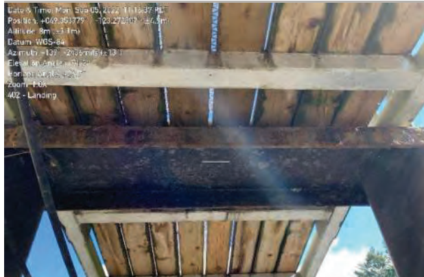
018. Minor Surface Corrosion of Pier Cap
