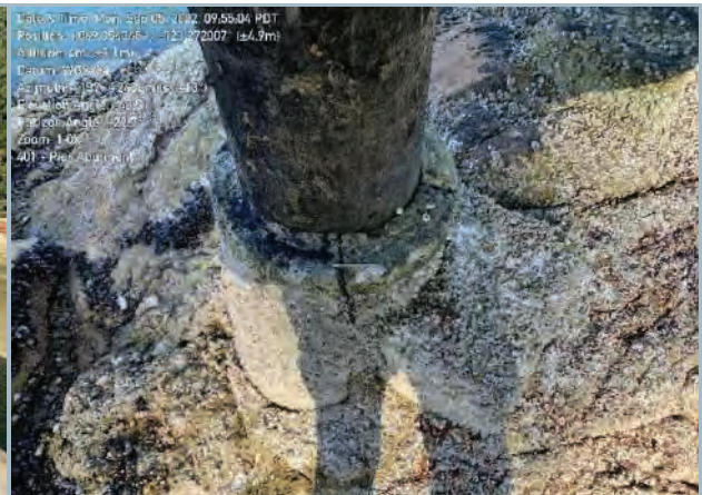
025. Cracked Concrete Pedestal at Bedrock Pier
