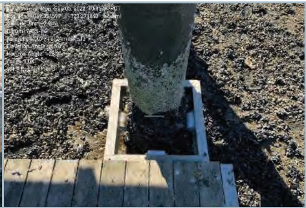
010. Dock Restraint Timber Pier Connection
