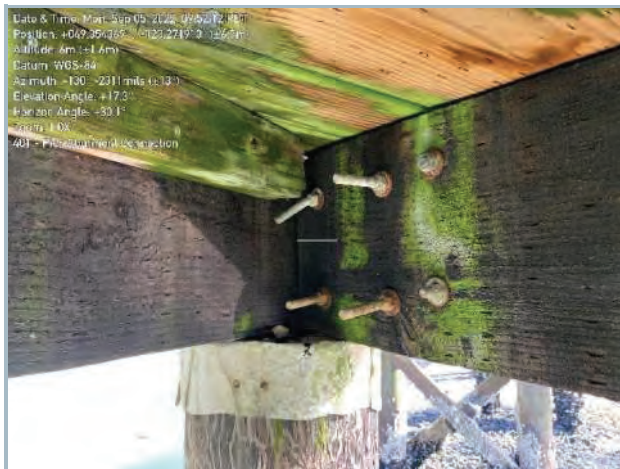
038. Inadequate Placement of Anchors at Bedrock Pier
