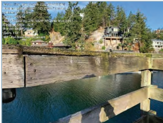
030. Localized Lifting of Decaying Top-rail, Typ.
