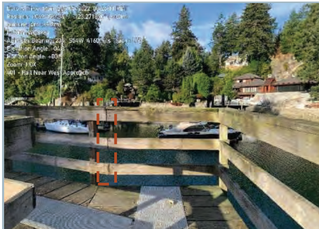
024. Vertically Unsupported Timber Splice at Bedrock Pier
