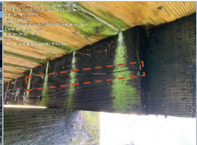
037. Full Longitudinal Splitting of Timber Splice
