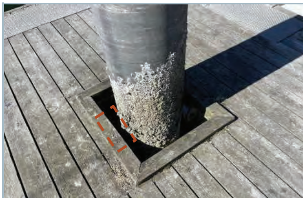
017. Timber Pile Dock Restraint System, Typ. (Note: Missing Roller Support)
