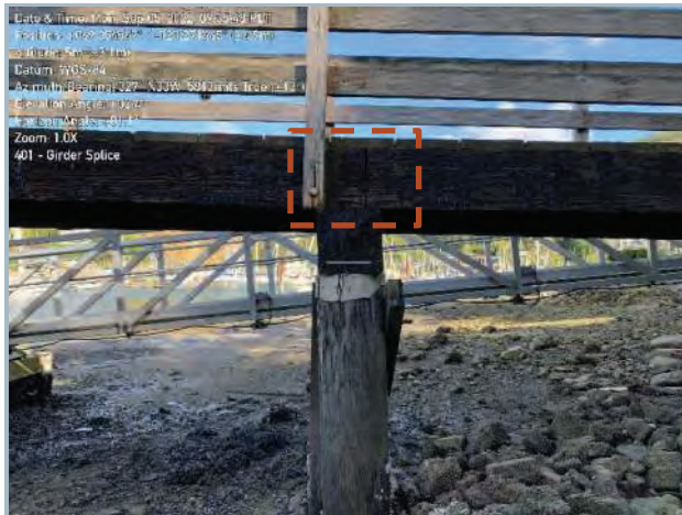
036. Unbalanced Longitudinal Beam Bearing Seat
