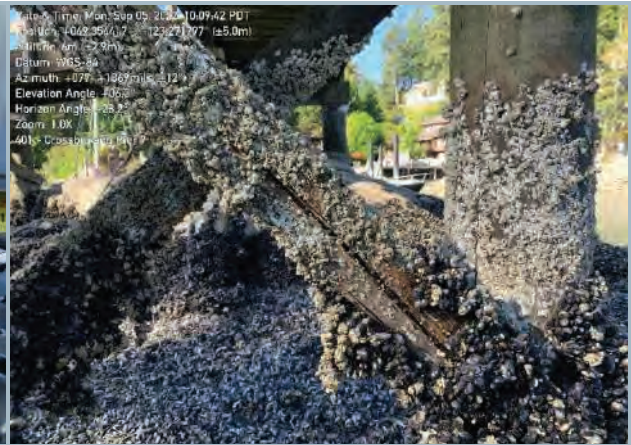
027. Decaying Timber Brace at Pier, Typ.
