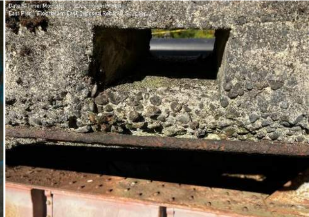
057. Concrete Spall and Exposed Reinforcing at Midspan of South Girder Profile
