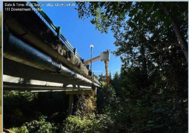
016. Utility Pipe Along South Profile
