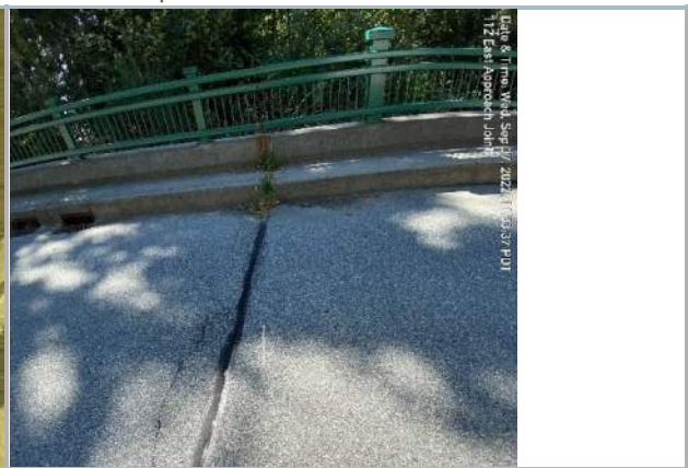
1021. Cracking of Asphalt Wearing Surface at East Approach Joint
