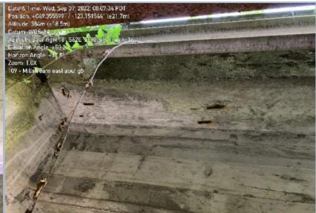
021. Exposed Reinforcing along Girder 1 (From North Profile)
