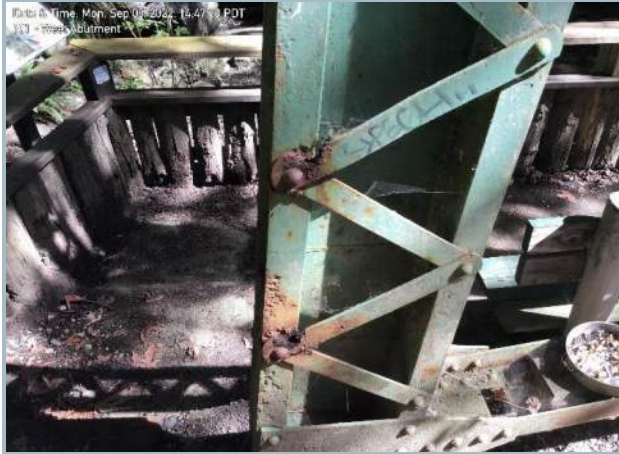
024. Pitting and Crevice Corrosion at West Pier Lattice, Typ.
