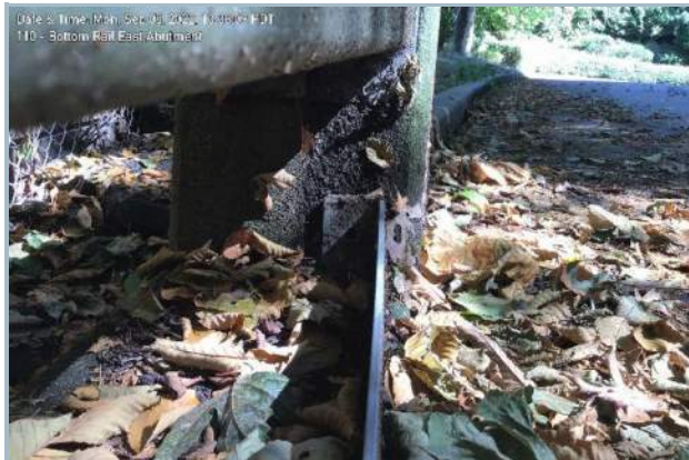
016. Dislodged Bottom Rail at Southeast Corner
