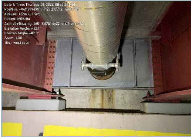
011. Central Waterman Utility (Note Staining of Backwall)
