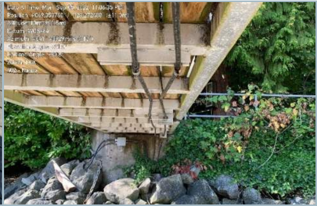
014. Electrical Utility Along North Profile of Deck Soffit
