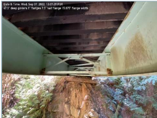
016. Lateral Bracing Members with Top Chord Diagonal Braces (Note: Birds Nest)
