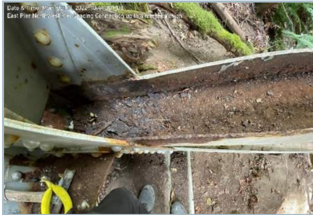
050. 4mm Section Loss at Northwest Base of West Pier
