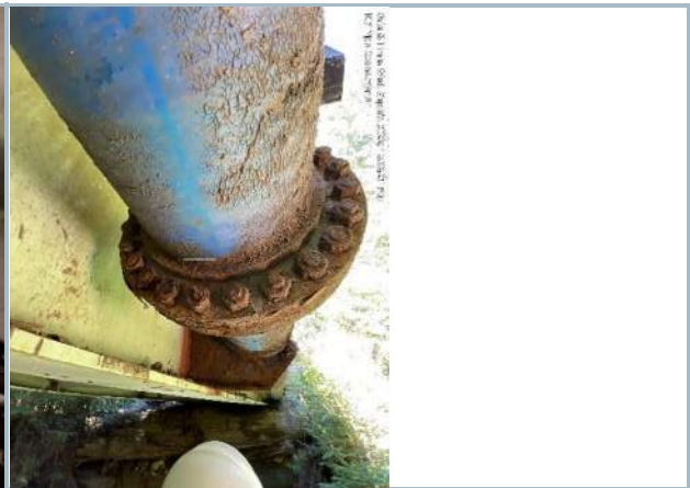
021. Corroding Utility Pipe Joint
