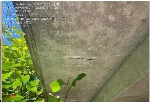
1017. Localized Exposed Reinforcing along North Profile
