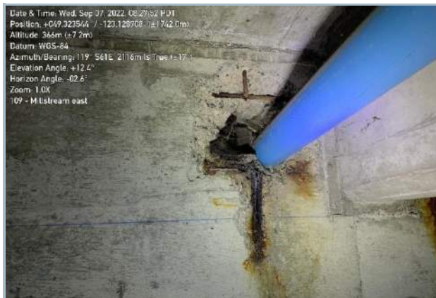
022. Concrete Spalling and Exposed Reinforcing at Utility Pipe Connection at East Abutment
