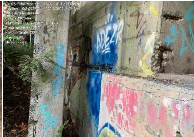
055. Exposed Reinforcing at South Wall of East Abutment
