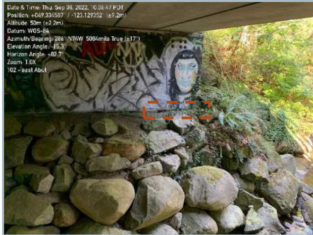
031. Undermining at Northwest Section of West Abutment
