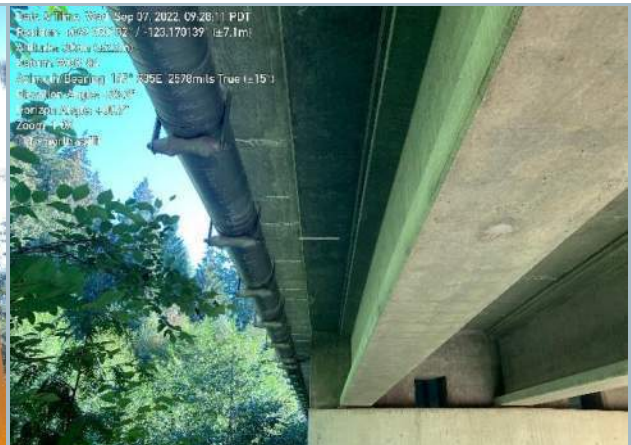
014. North Profile Overhang Soffit (Note Intermittent Efflorescence)
