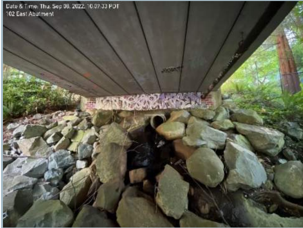
007. East Abutment (Note Storm Sewer Outfall)
