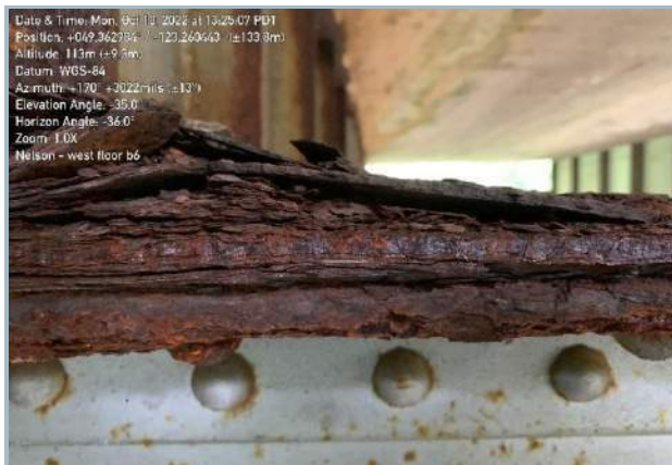
040. Accelerated Uniform Corrosion on Top Flange of Floor Beam 5, Typ.
