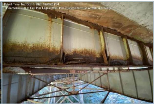
039. 3-5mm Section Loss on Bottom Flange of Floor Beam 9 (Note: Top Flange Corrosion, Typ.)
