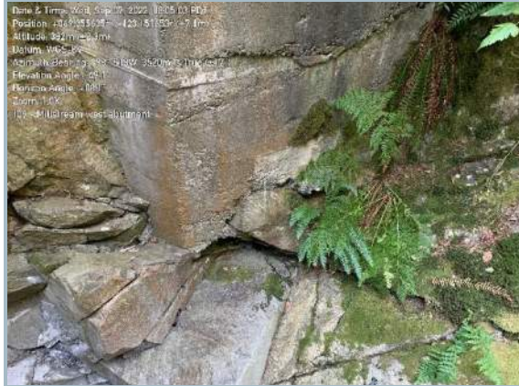
024. Undermining at South Section of West Abutment
