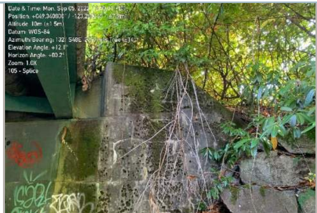
025. Efflorescence and Cracking at Southeast Wingwall
