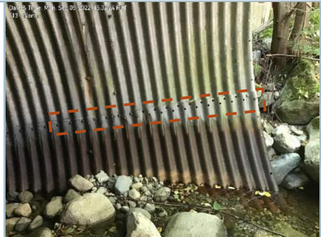
014. Missing Splice Bolts at Inlet
