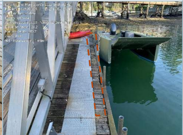
033. Decay Deck Members at East Profile of Dock
