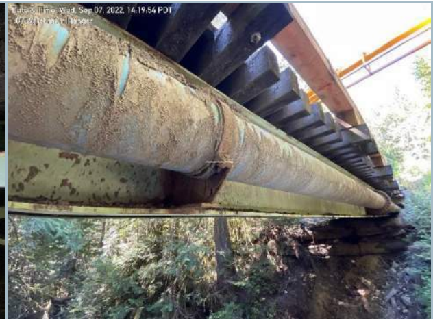
025. Corroding Pipe Hanger, Typ.
