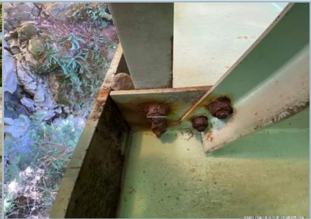
023. Degrading Bolts at Cross-brace Gusset Plate
