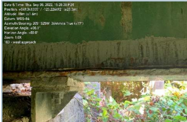
025. Bottom Flange Surface Corrosion and Deposit Attack at Abutment, Typ.
