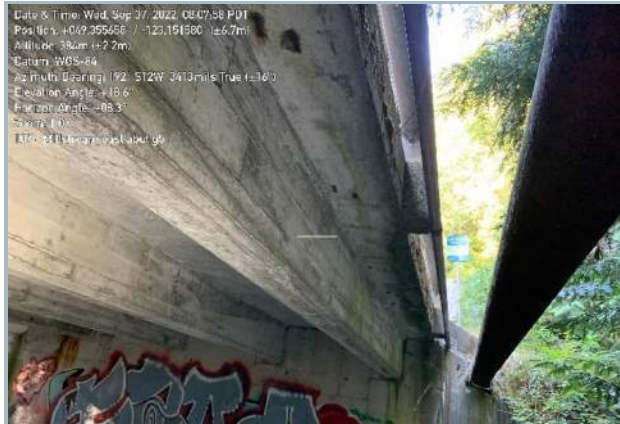
024. Staining of Deck Soffit at Southmost Girder
