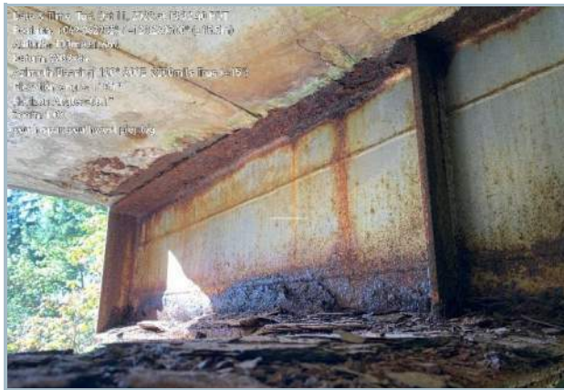
038. Accelerated Uniform Corrosion at Bottom Flange of Floor Beam 5
