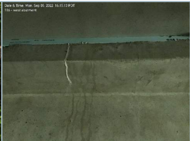
020. Minor Cracking & Efflorescence along Top Flange of Central Girder at West Abutment
