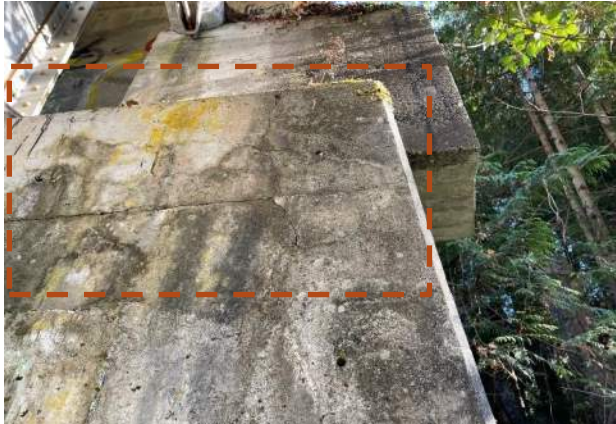
062. Extensive Cracking at East Abutment Side Wall
