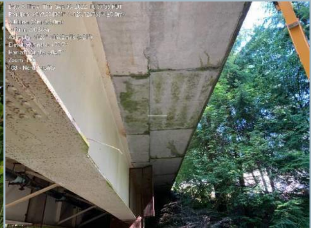
020. Sidewalk Soffit along East Profile, Typ.
