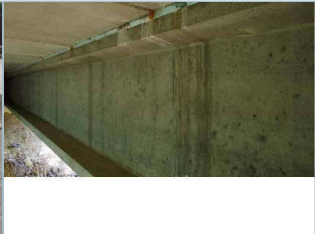
018. Moisture Ingress at Soffit Below Cracked Asphalt of Approach Slab
