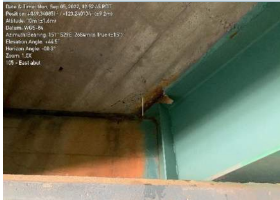
028. Top Flange Corrosion and Concrete Delamination at Soffit, Typ.
