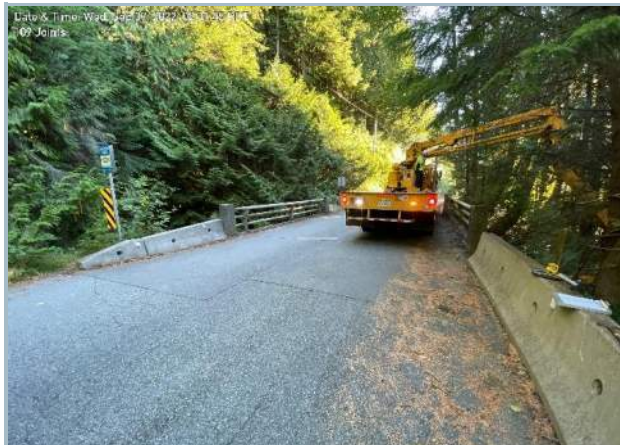
015. West Approach Slab Joint
