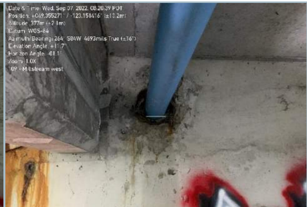
027. Spalling and Staining Around Gas Utility Line at West Abutment
