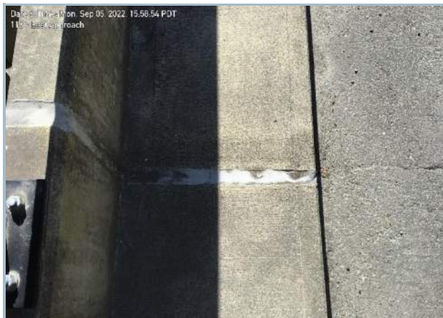
014. Non-continuous Joint Application for Approach Slab
