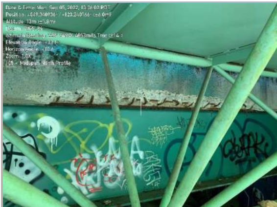
024. Exposed Section of Reinforcing at North Profile, Typ.
