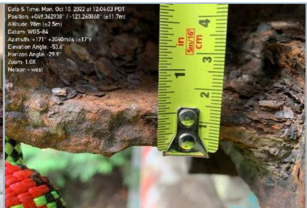
041. 3-5 Section Loss at Bottom Flange of Floor Beam 5 Below Expansion Joint
