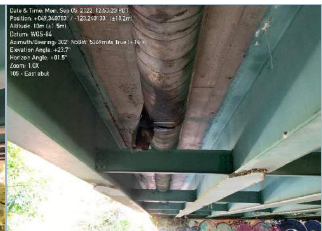
017. Watermain Utility Along South Profile (Note: Deterioration of Pipe Surface at Midspan)
