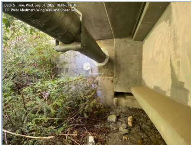
019. Elastomeric Bearing at North Section of East Abutment (Note: Elastomeric Pad on Short Side Wall Restraint)
