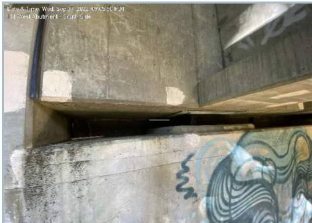
107. Elastomeric Bearing at South Section of West Abutment (Note: Elastomeric Pad on Short Side Wall Restraint)
