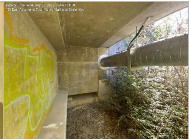
020. Elastomeric Bearing at South Section of East Abutment (Note: Elastomeric Pad on Short Side Wall Restraint)
