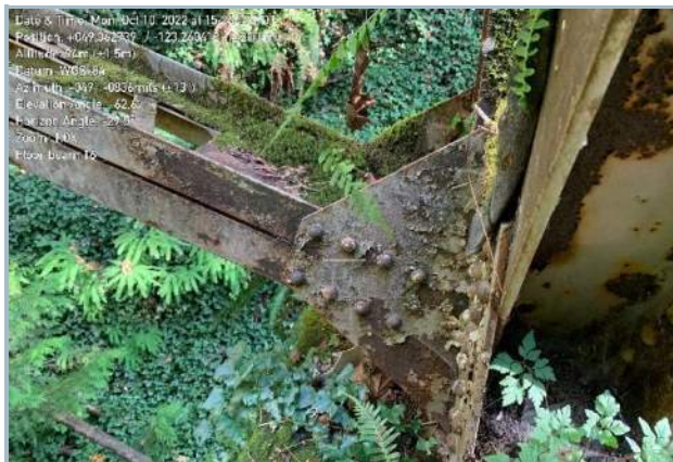
052. Vegetation Growth on East Pier Connection, Typ.
