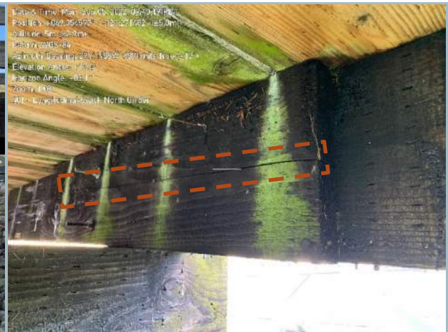
037. Full Longitudinal Splitting of Timber Splice
