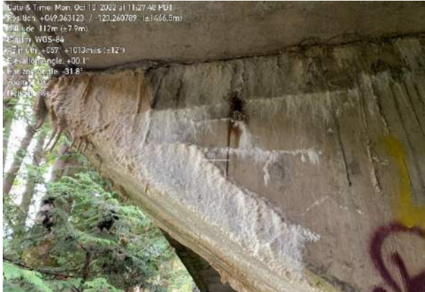
060. Efflorescence on Deck Soffit of West Abutment
