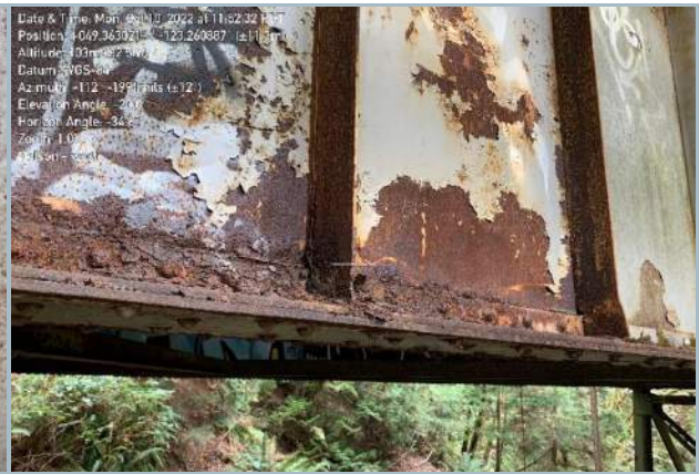
037. Deposit Attack and Accumulation on Bottom Flange of South Girder, Typ. (Note: Deterioration of Rivets)
