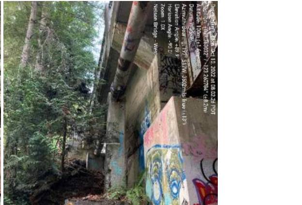
065. Undermining and Aggregate Exposure West Abutment Wing Wall
