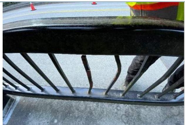
018. Dislodged Picket at Northwest Section
