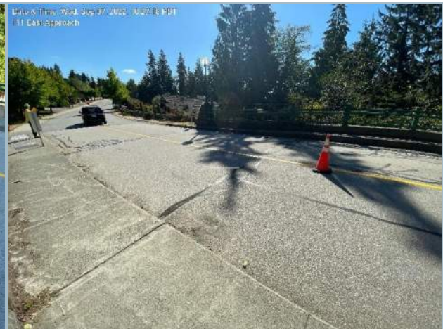
014. East Approach Slab Joint
