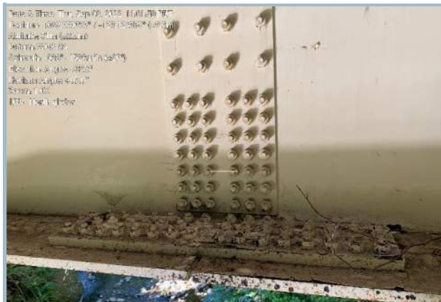
017. Localized Sections of Coating Failure at Splice Locations, Typ.
