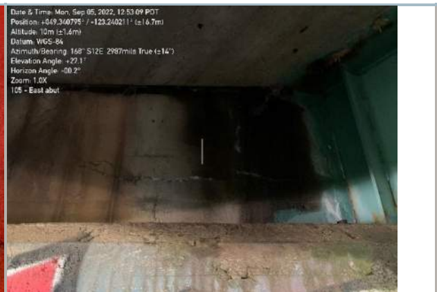
027. Efflorescence and Cracking at East Abutment Back Wall, Typ.
