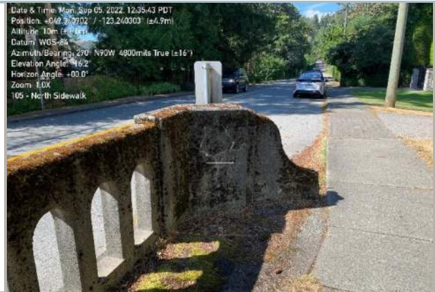
023. Efflorescence and Cracking Northwest Section of Parapet
