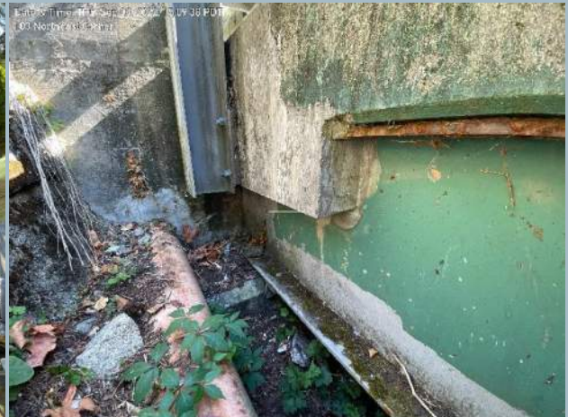
016. Sanitary Utility Connection at East Abutment
