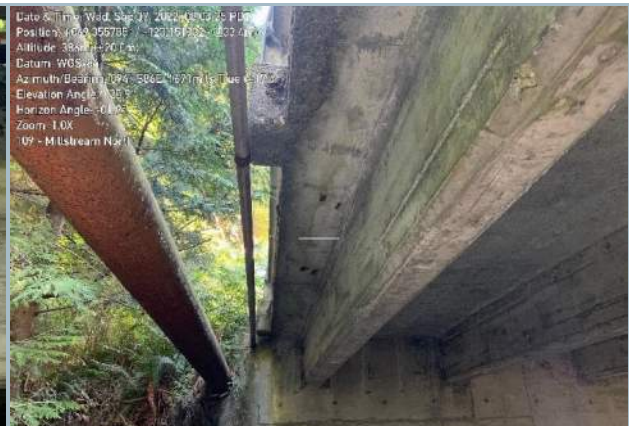
019. Exposed Reinforcing along Girder 1 Soffit (Northmost Girder)
