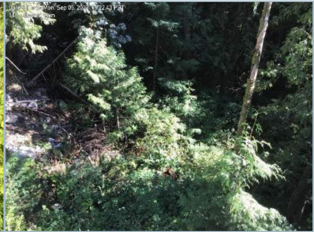
002. Downstream (Note Extensive Vegetation Growth and Poor Slope Stability)
