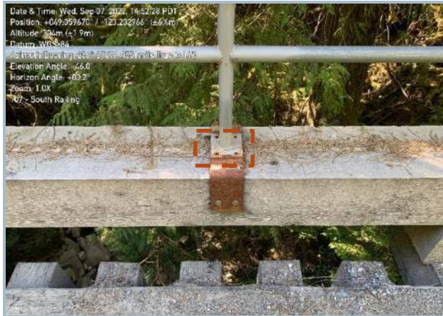
022. Anchor Bolts Not Installed at Rail Connection
