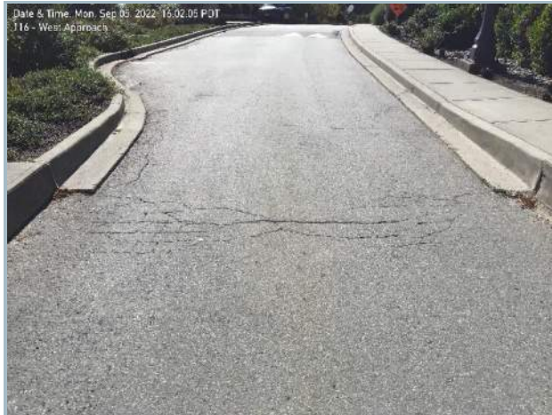
017. Cracking of Asphalt Wearing Surface Along Approach Slab, Typ.
