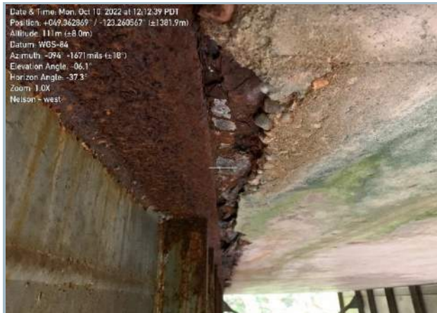
046. Top Flange Corrosion and Spalling of Deck Soffit at Floor Beam 14
