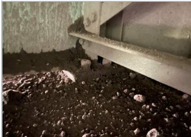
020. Debris Accumulation at Bearing Plate, Typ.
