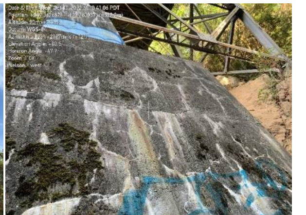
059. Extensive Efflorescence at Southeast Pedestal of West Pier
