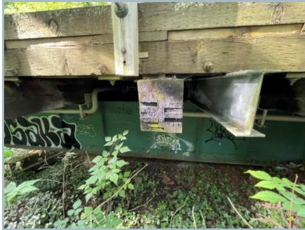
013. Retrofit Installation of Transverse Steel Elements Bearing on Riveted Steel Plate Girders
