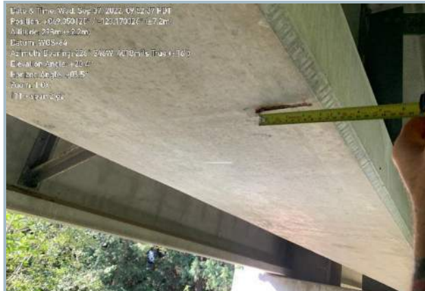
025. Localized Exposed Reinforcing at Midspan of Central Girder (Adjacent to West Pier)
