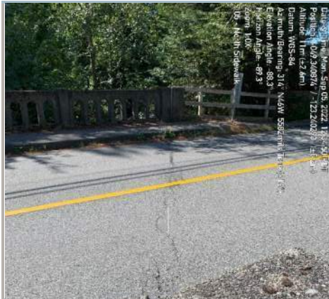
022. Cracking in Asphalt Wearing Surface of West Approach Slab
