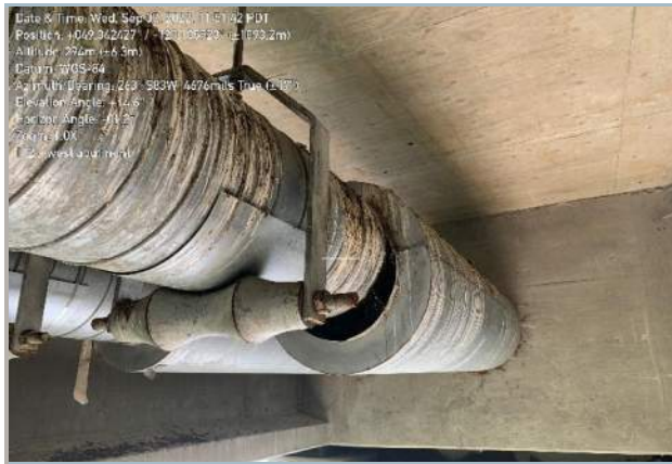
1016. Void at Utility Pipe Connection
