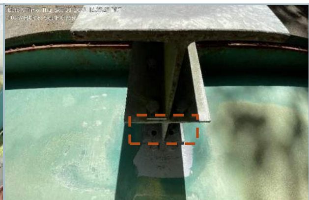
028. Railing Support Connection Bolts Missing Along South Profile, Typ.
