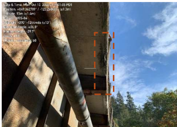
058. Localized Sections of Exposed Reinforcing at Midspan along South Profile, Typ.
