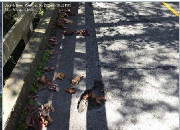
029. Cracking on Asphalt Wearing Surface, Typ.
