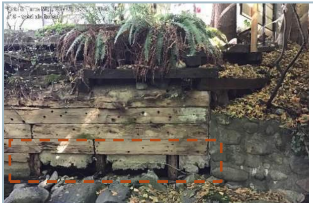
018. Degrading Timber Retaining Wall at Northeast Corner
