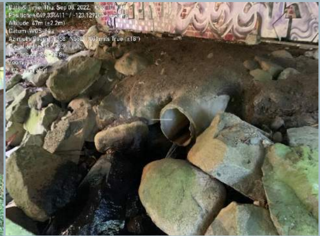
014. Stormwater Outfall at East Abutment (Note Scouring)
