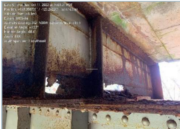
042. Complete Section Loss at Floor Beam 7
