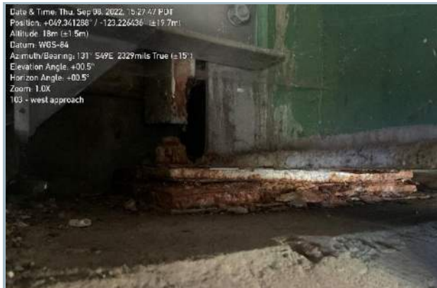
023. Corrosion-led Delamination of Steel Bearing Plate, Typ.
