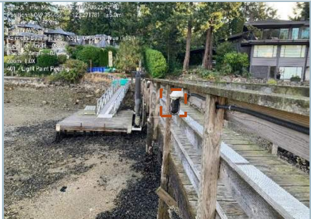
029. Diminishing Black Paint on Light Fixtures, Typ.
