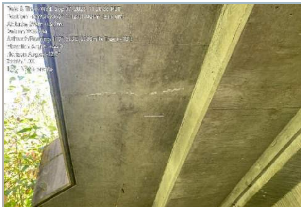
1020. Minor Efflorescence at North Profile
