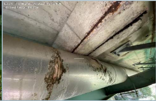
030. Exposed Reinforcing on Concrete Soffit (Note Localized Deterioration of Pipe Surface)
