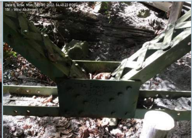
027. Debris accumulation at Pier Connections, Typ.
