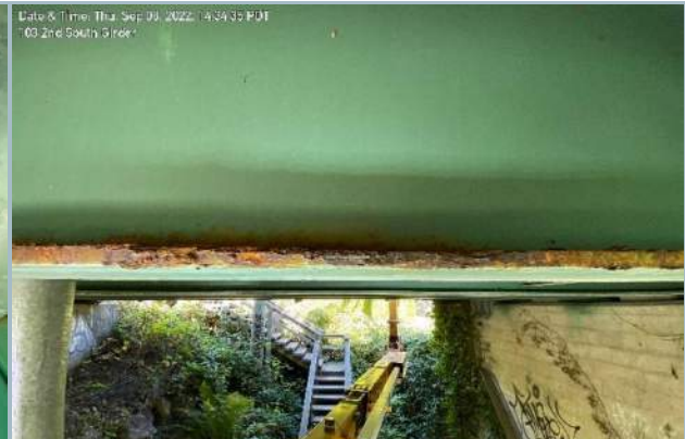
032. Localized Corrosion-led Deterioration of Bottom Flange at West Pier, Typ.
