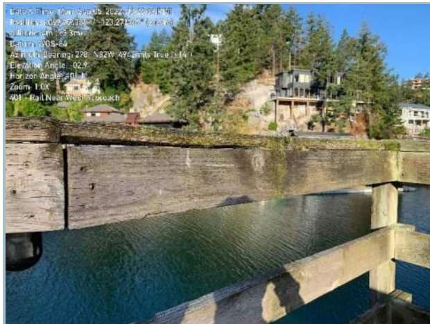
030. Localized Lifting of Decaying Top-rail, Typ.
