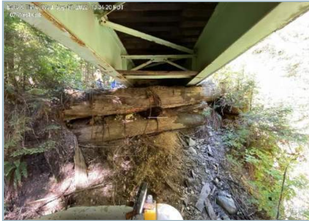
018. Unsecure Timber Crib at North Abutment
