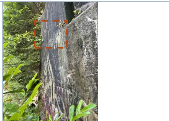
033. Wingwall Cracking at Southwest Side Wall
