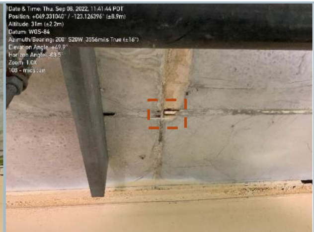
022. Localized Sections of Exposed Reinforcing along Deck Soffit
