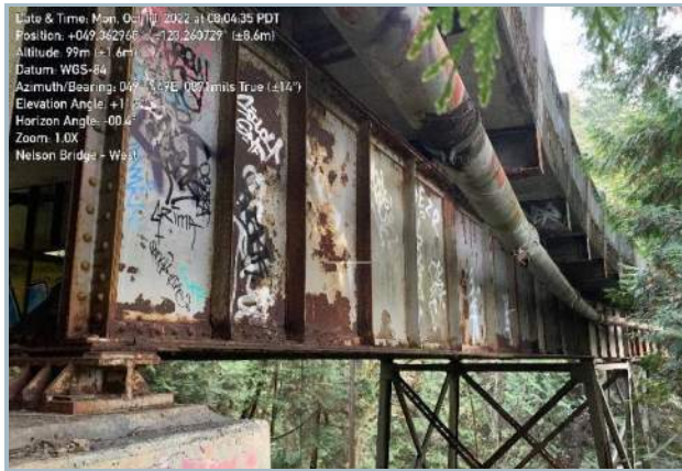
048. South Girder Bottom Flange Corrosion, Typ.
