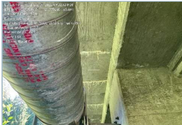
023. Intermitting Efflorescence along Overhang Soffit of North Profile
