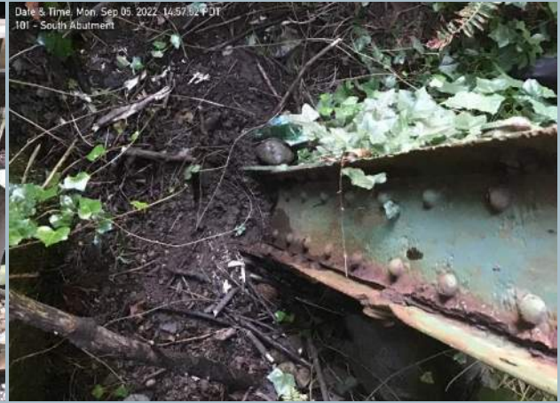
025. Buried Southeast Pier Footing (Note Corrosion-led steel delamination)
