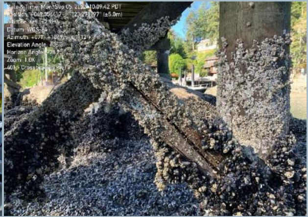
027. Decaying Timber Brace at Pier, Typ.
