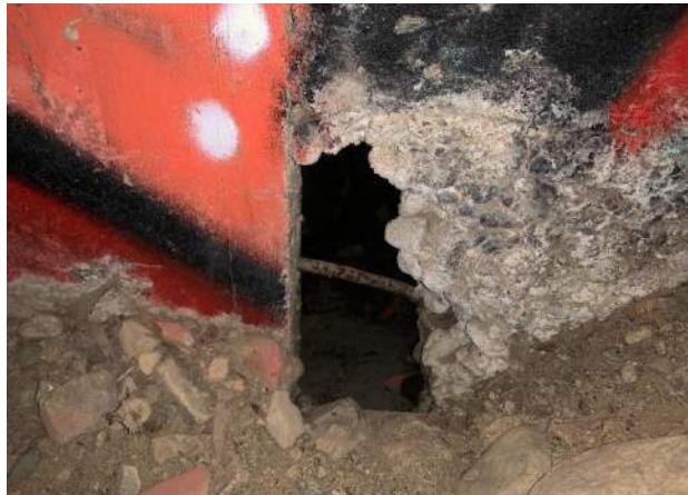
054. Concrete Void at West Abutment South Side Wall
