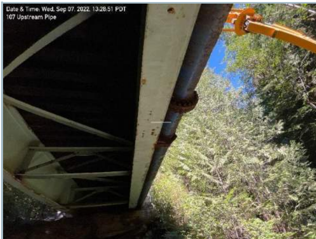
026. Intermittent Under Film Corrosion on Bottom Flange of West Girder
