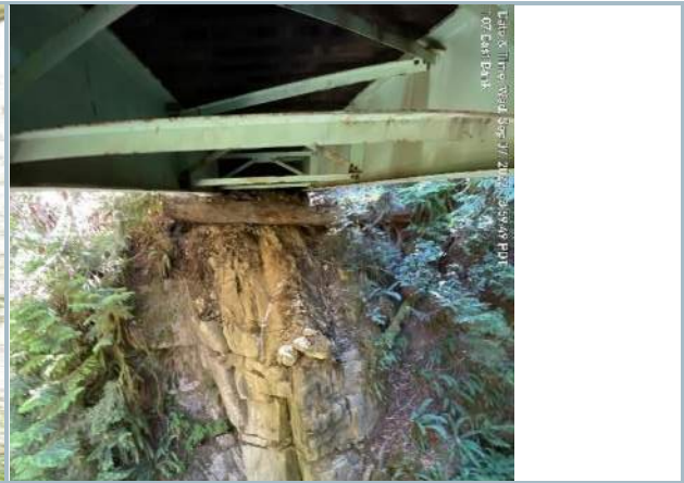
019. Unsecure Timber Crib at South Abutment
