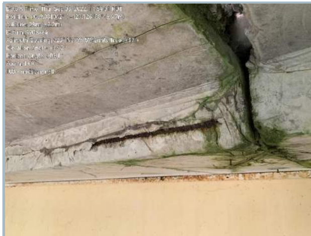
021. Exposed Reinforcing Adjacent to Deck Joint Separation (Note Extensive Cracking Emanating from Deck Joint)
