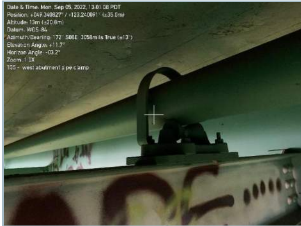
018. Gas Pipeline Support, Typ.
