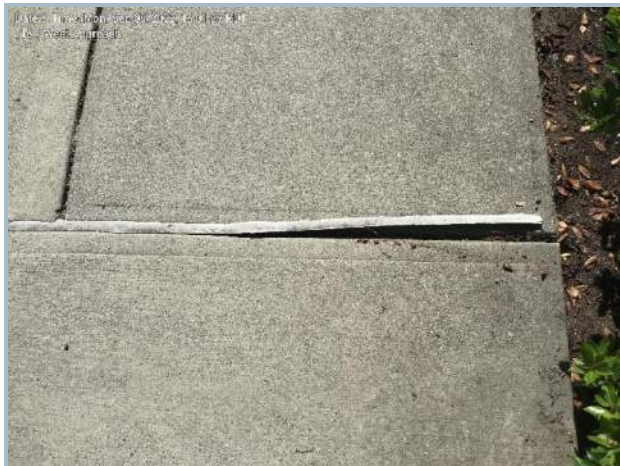
019. Expansion Joint Peel at Northeast Section of Sidewalk
