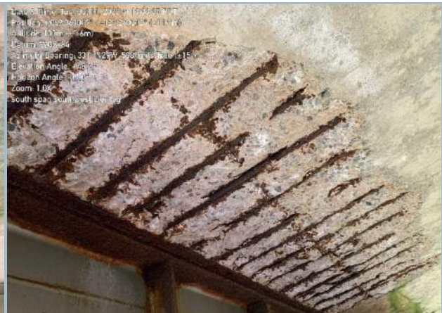
047. Exposed Reinforcing Section of Deck Soffit at Floor Beam 15
