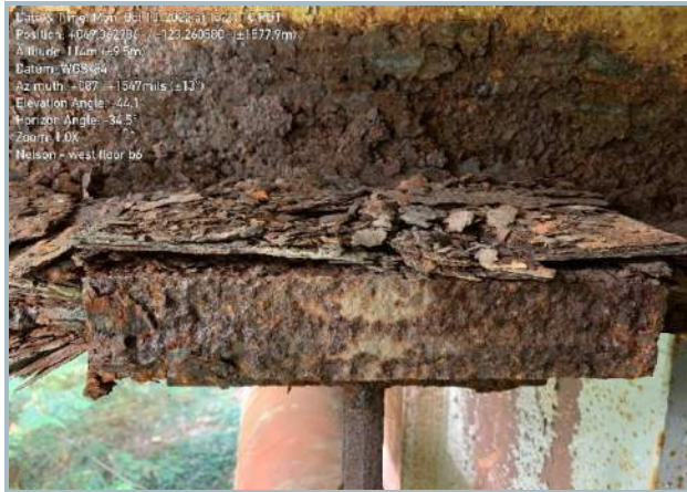
044. Accelerated Uniform Corrosion at Bottom Flange of Floor Beam 6
