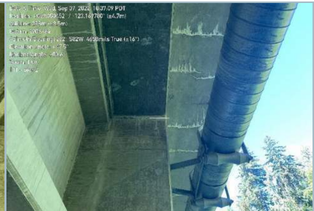
024. Intermitting Efflorescence along Overhang Soffit of South Profile
