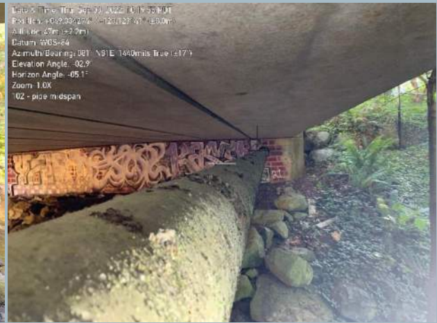
032. Vegetation Growth and Localized Corrosion of Watermain Utility
