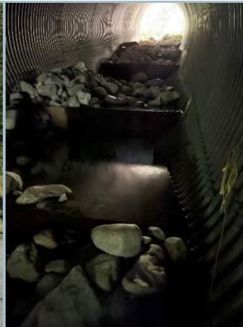
012. Culvert Interior (Note Obstructed Baffles)
