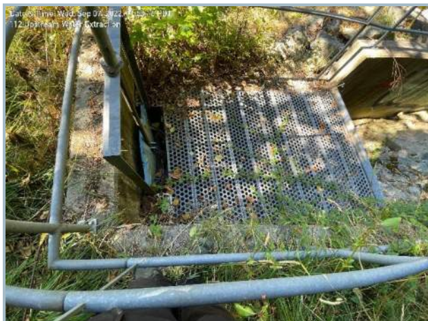
017. Upstream Water Extraction System
