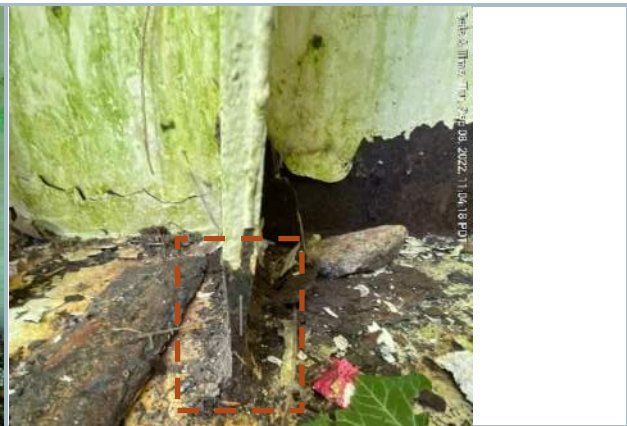
014. Stiffener Section Loss at Southwest Corner
