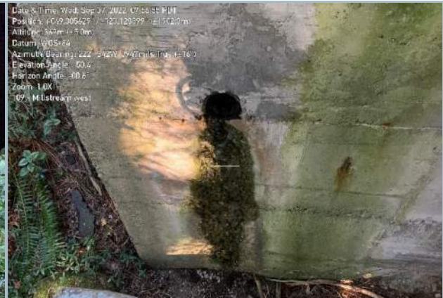
025. Spalling and Staining of Drain Outlet at West Abutment
