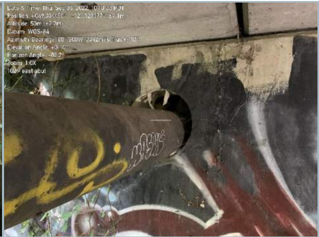
028. Void around Watermain Utility at West Abutment (Note: Utility Pipe Directly bearing on Backwall)
