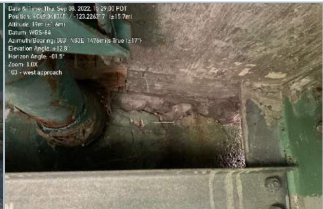
024. Concrete Delamination & Cracking Adjacent to Pipe Connection at West Abutment (Note: Bolted Lateral Restraint Connection)
