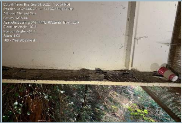
016. Localized Sections of Coating Failure at Bottom Flange of South Girder, Typ.
