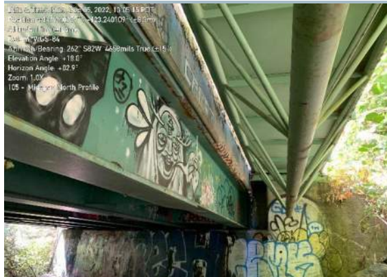
030. Continuous Top Flange Corrosion of North Stringer, Typ.
