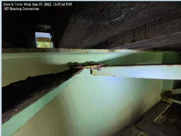
024. Degrading Bolts on Gusset Plate Connection Subject to Crevice Corrosion
