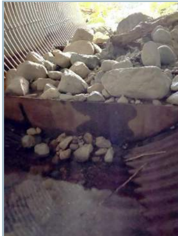
013. Obstructed Bulkheads, Typ.
