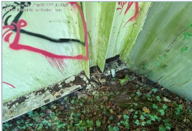
023. Coating Failure on Bottom Flange of Girder at Southwest Corner
