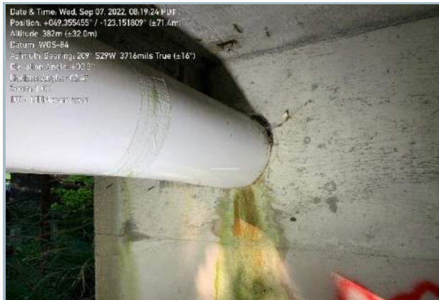
026. Staining of Utility Line at West Abutment
