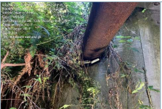
029. Spalling and Staining of Utility Line Connection at Northeast Wing Wall
