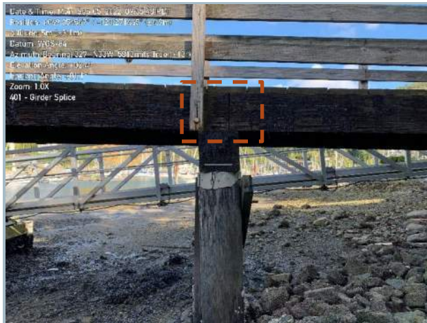
036. Unbalanced Longitudinal Beam Bearing Seat
