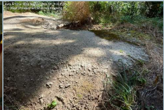
026. Cracking of Shotcrete on West Embankment
