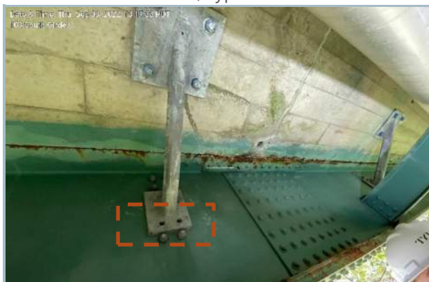
027. Railing Support Connection Bolts Missing Along South Profile, Typ. (Note Continuous Top Flange Corrosion, Typ.)
