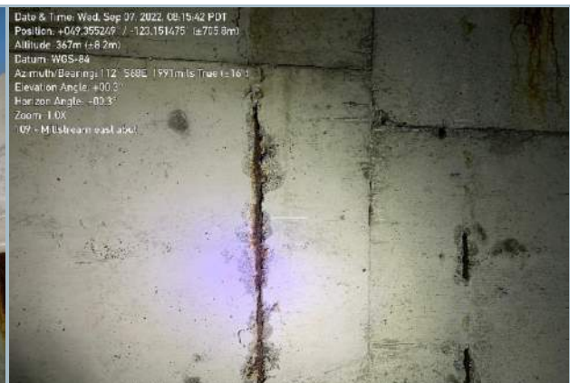
023. Exposed Reinforcing at East Abutment
