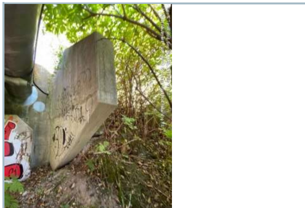
027. Wing Wall at Northwest Section Not Retaining Fill
