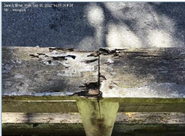
028. Decaying Timber Rail and Curb Components
