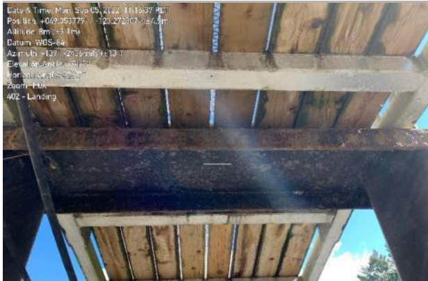
018. Minor Surface Corrosion of Pier Cap
