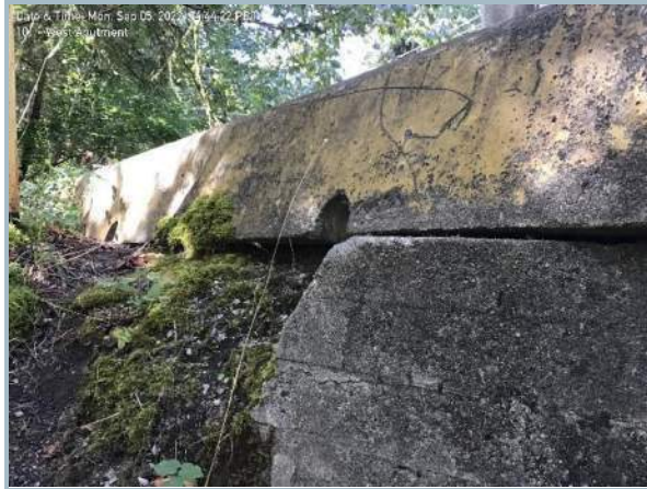
015. Barrier Bearing on Southwest Wingwall (Note Minor Undermining)
