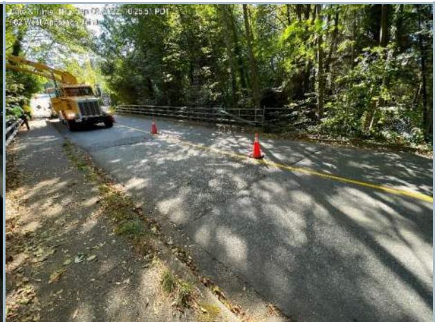
030. Cracking of Asphalt Wearing on West Approach Indicating Probable Settlement
