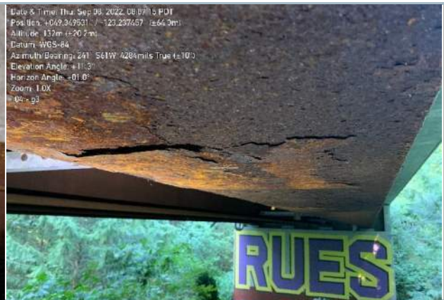
014. Localized Mill Scale Flaking on Bottom Flange of Weathering Steel (Expected Behavior)
