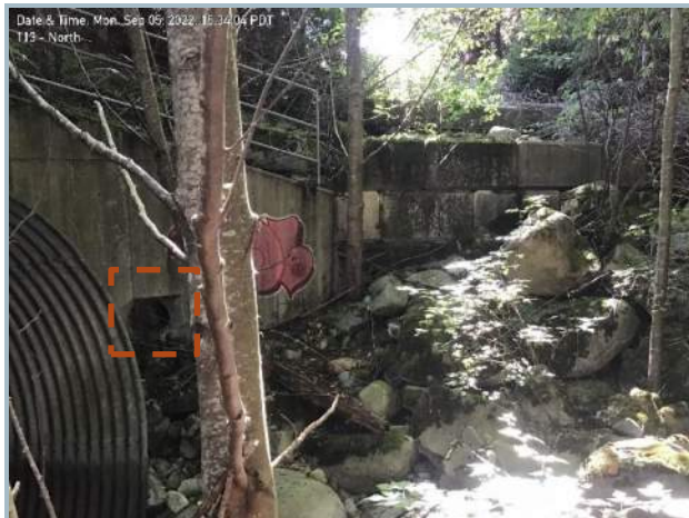
015. Stormwater Outfall West of Culvert Inlet
