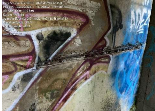
056. Exposed Reinforcing at South Section of West Abutment Side Wall
