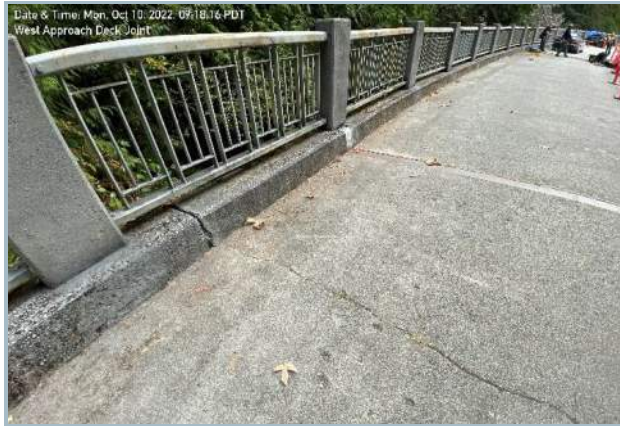
066. Cracking on Asphalt Wearing Surface at West Approach Deck Joint, Typ.
