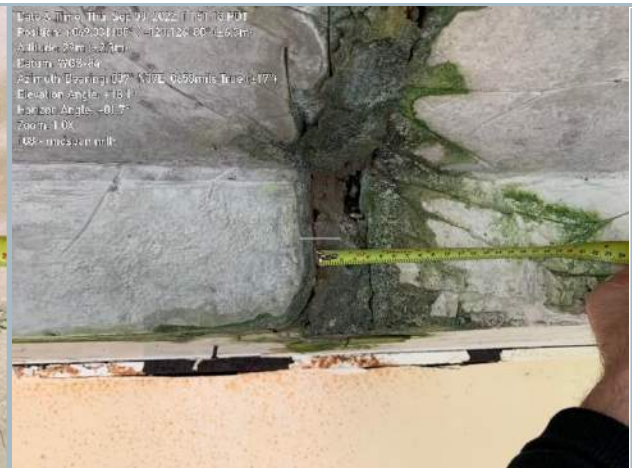
020. 1.5" Concrete Void at Deck Joint Viewed Along East Profile
