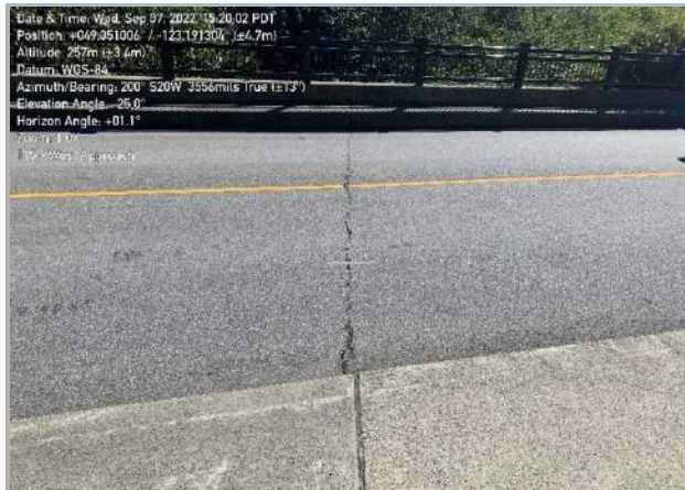
021. Cracking of Asphalt Wearing Surface at West Approach (Note Skewed Orientation)
