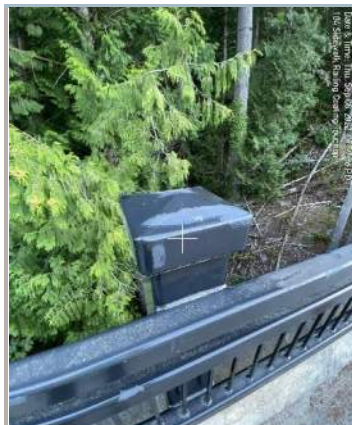
017. Minor Discolouration in Rail Coating
