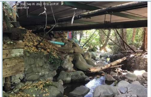
017. Debris Accumulation Within Channel
