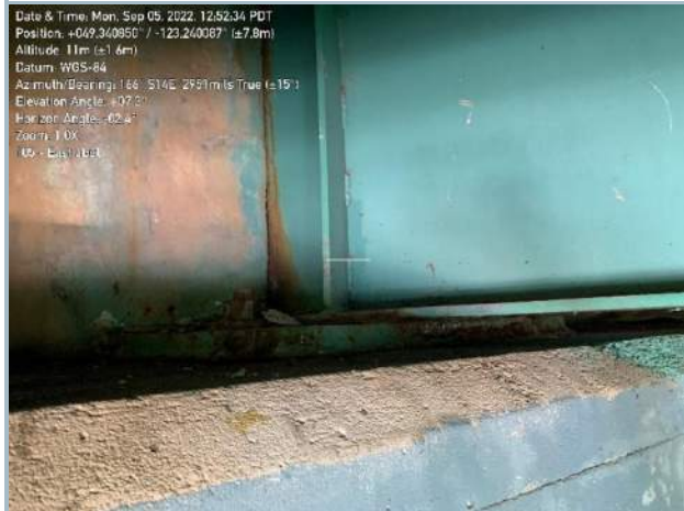
020. Anchored Steel Bearing Plate, Typ. (Note Surface Corrosion)
