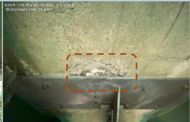
026. Spalling above East Pier Brace
