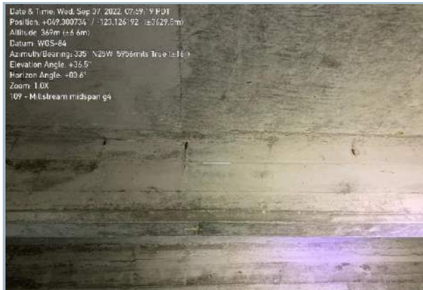
020. Exposed Reinforcing along Girder 2 (From North Profile)
