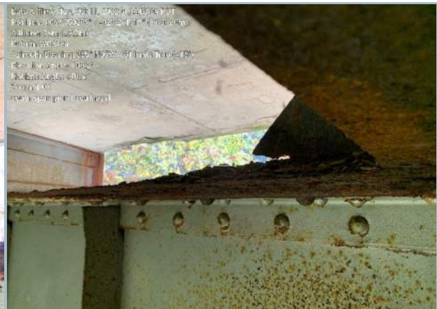
043. Steel Delamination and Deposit Accumulation at South Girder, Typ.
