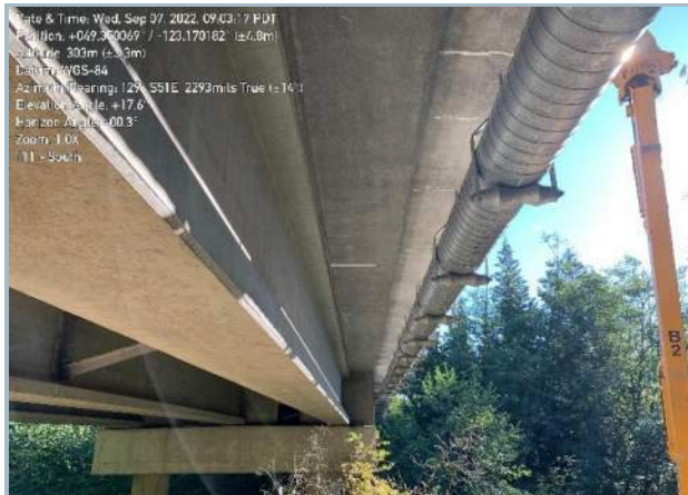
013. South Profile Overhang Soffit (Note Intermittent Efflorescence)
