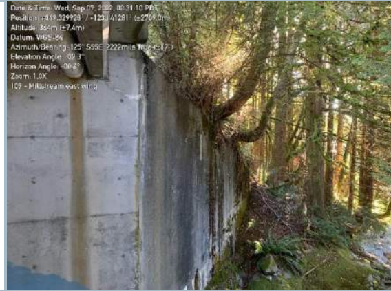
025. Excessive Vegetation Supported by Wing Wall
