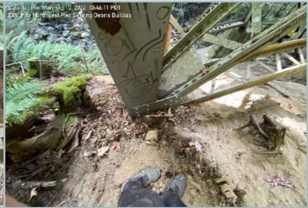
051. Debris Accumulation at Pier Northwest Column Base of East Pier
