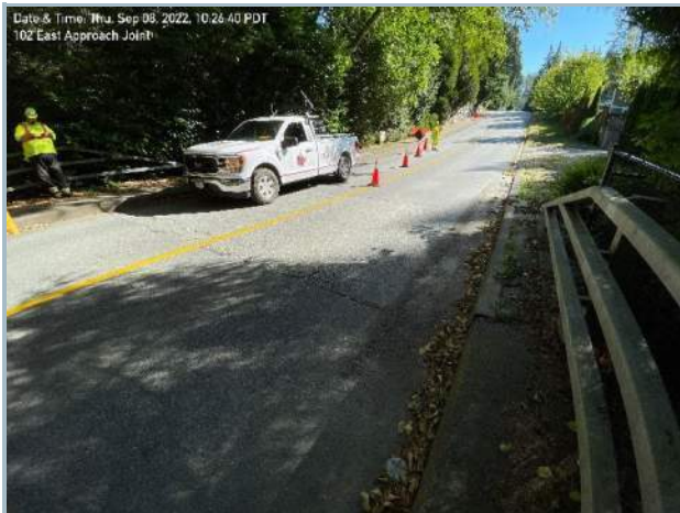
029. Cracking of Asphalt Wearing on East Approach Indicating Probable Settlement
