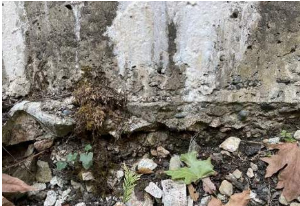
064. Undermining and Aggregate Exposure East Abutment Wing Wall
