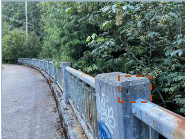
068. Localized Exposed Reinforcing on Deck Parapet at Midspan
