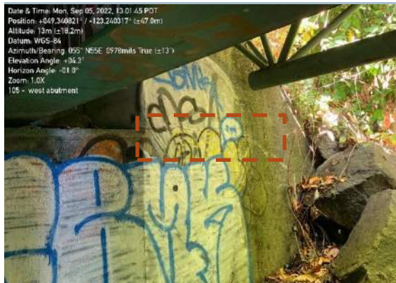
032. Cracking at Northwest Wingwall Section
