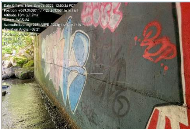
026. Longitudinal Cold-joint Separation at East Abutment Front Wall
