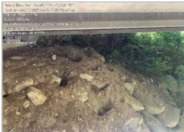
023. Scour Accumulation on West Embankment
