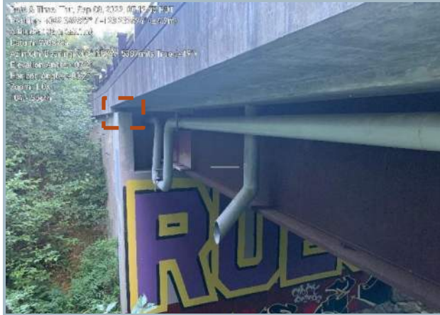
013. Retaining Wall Separation (Note Utility Line Along South Profile)
