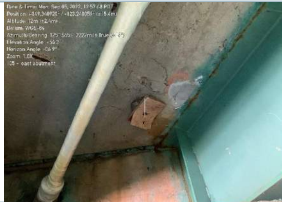
029. Localized Exposed Reinforcing at Soffit, Typ. (Note: Concrete Delamination at Northeast Section of East Abutment)
