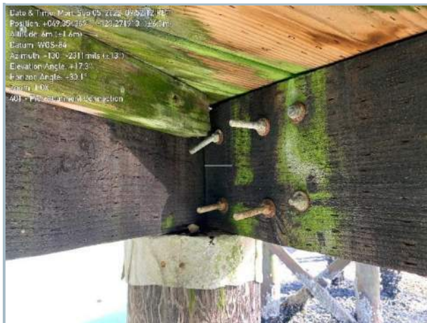
038. Inadequate Placement of Anchors at Bedrock Pier
