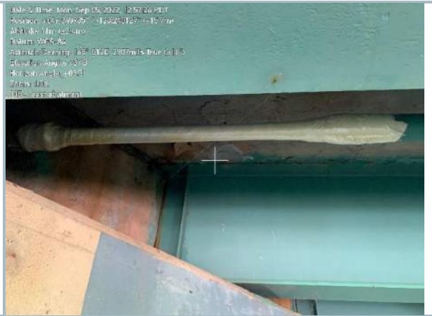
019. Gas Utility Pipe Diameter Transition at North Profile
