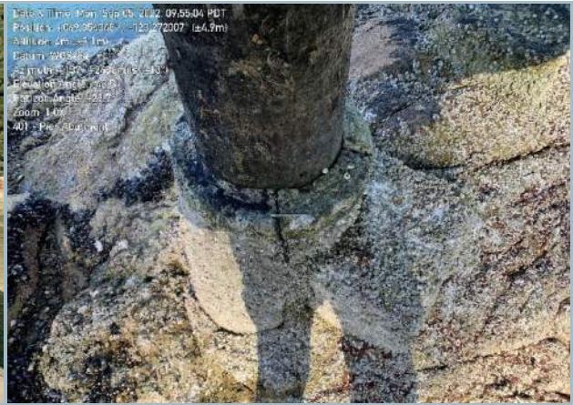
025. Cracked Concrete Pedestal at Bedrock Pier
