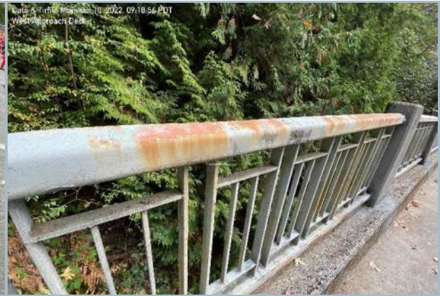
067. Localized Inconsequential Surface Corrosion on Northwest Railing, Typ.
