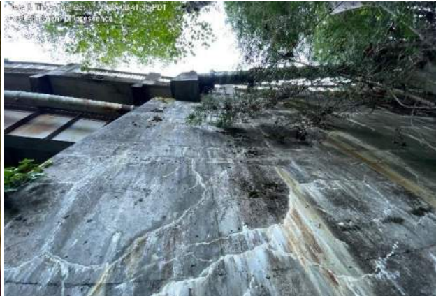
061. Extensive Efflorescence at East Abutment Wing Wall
