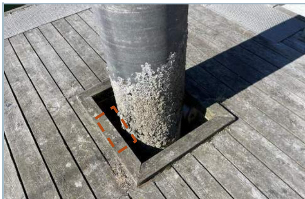
017. Timber Pile Dock Restraint System, Typ. (Note: Missing Roller Support)
