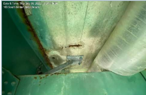
031. Exposed Reinforcing on Concrete Soffit at Midspan along Second Girder from South Profile (Note: Efflorescence and Cracking around Previous Deck Drain)
