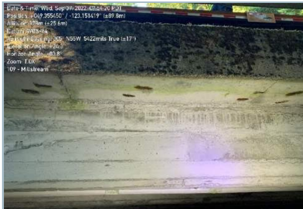
018. Exposed Reinforcing along Girder 5 Soffit (Southmost Girder)
