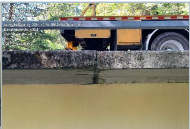
018. Separation in Concrete and Spalling Occurring at Deck Joints, Typ.
