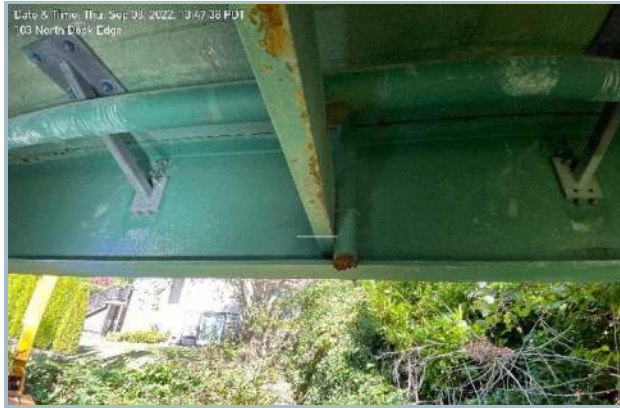
029. Corroding Drainpipe Outlets
