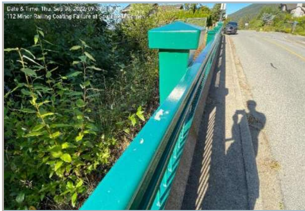
1018. Minor Coating Failure on South Railing
