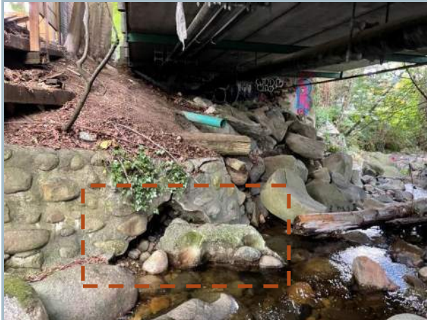
013. Utility Configuration Supported by Bridge (Note Dislodged Retaining Wall Section)
