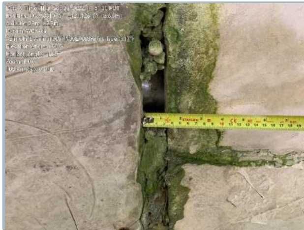
019. 1.25" Concrete Void at Deck Joint Viewed from Sidewalk Soffit
