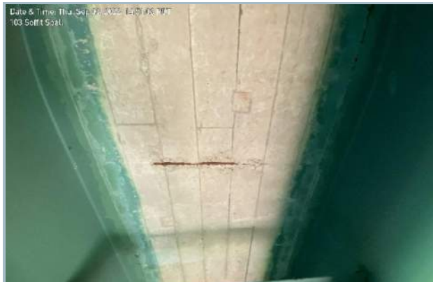
033. Exposed Reinforcing on Concrete Soffit at Midspan along South Profile
