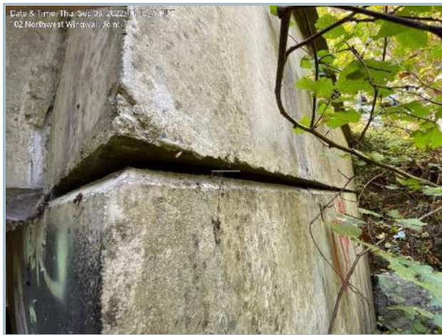
033. Notable Separation at Wingwall, Typ.
