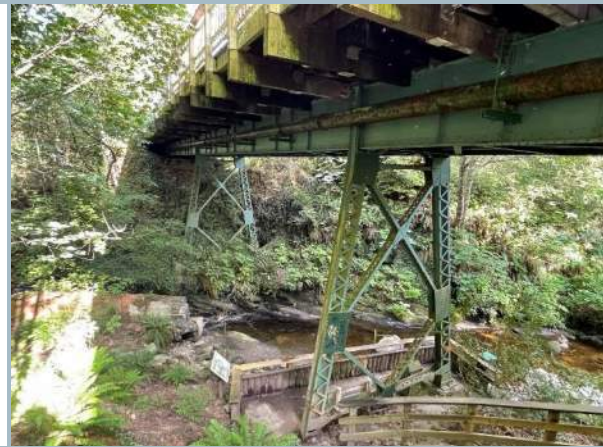
016. Watermain Utility along North Elevation (Note: Surface Corrosion of Pipe)
