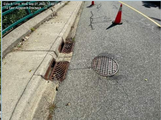
014. Stormwater Drainage on Deck, Typ.
