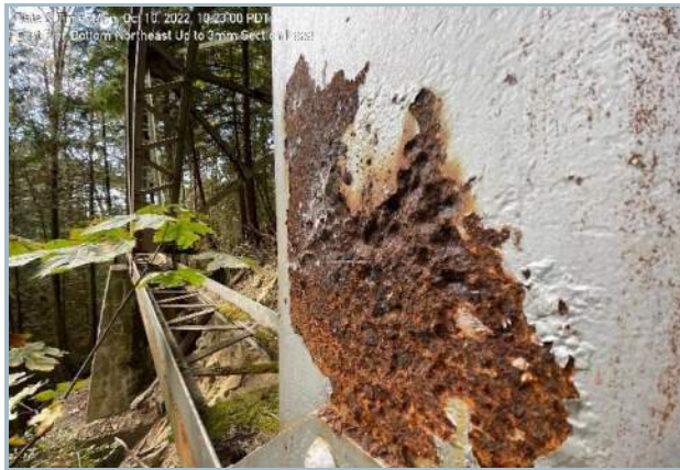
036. Pitting Corrosion with ~3mm Section Loss at Bottom of Northeast Pier
