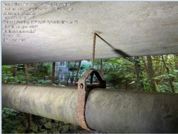
027. Corroding Pipe Hanger Support, Typ.
