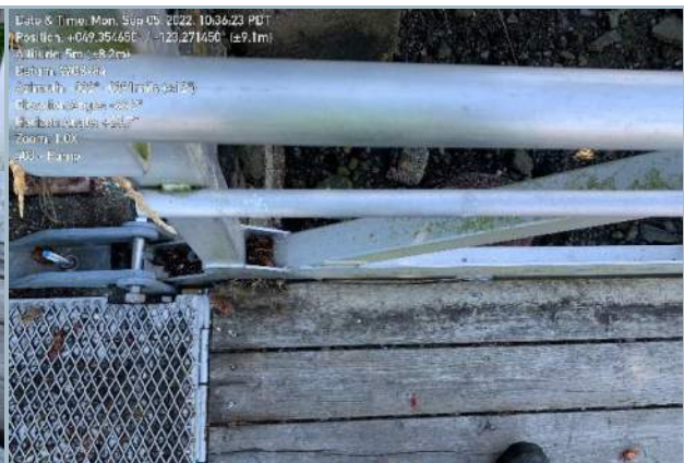
012. Debris Accumulation at Rail Truss Base
