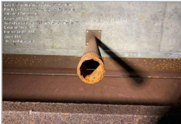
013. Corroding Weeping Drain Outlet, Typ.
