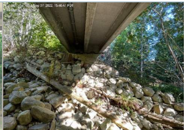
024. Debris Accumulation on East Embankment
