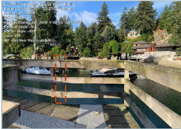
024. Vertically Unsupported Timber Splice at Bedrock Pier
