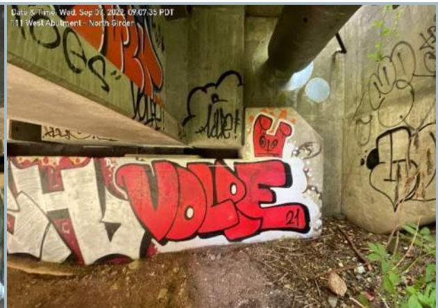
108. Elastomeric Bearing at North Section of West Abutment (Note: Elastomeric Pad on Short Side Wall Restraint)
