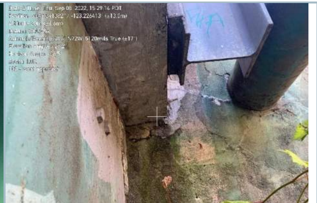
034. Cracking of Backwall around Sanitary Utility and Concrete Repair at West Abutment
