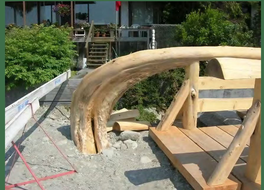
Bridge built with salvaged urban wood at the Lawson Creek Estuary in Ambleside
