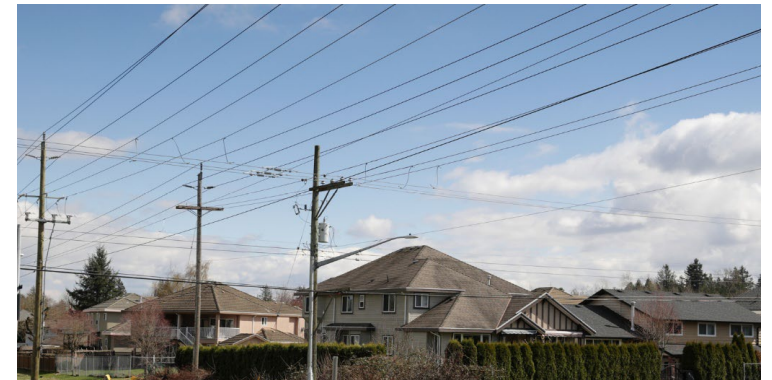
BCHydro.com – Power lines
