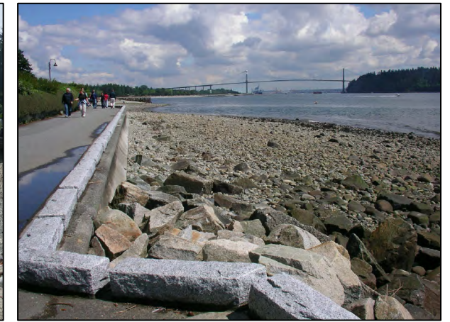
Photo 4. Example of vertical seawall, boulder softened shoreline, and bare substrate. Moderate productivity zone visible near waterline.
